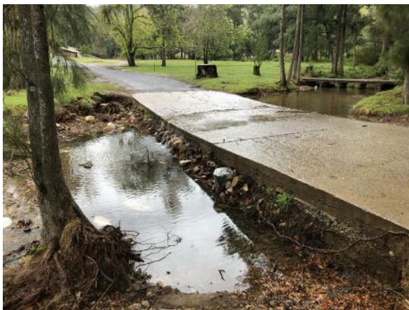
Reach B dropdown erosion at ford 30/9/21
