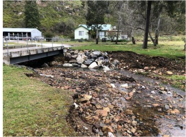
Reach B outer bed erosion and rock armour 30/9/21
