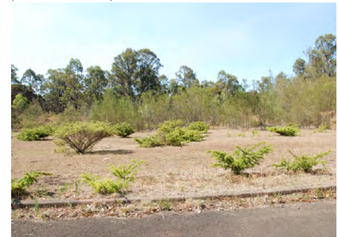
Site image: Kerb and gutters to Main Visitor Precinct (Source: EP NSW)
