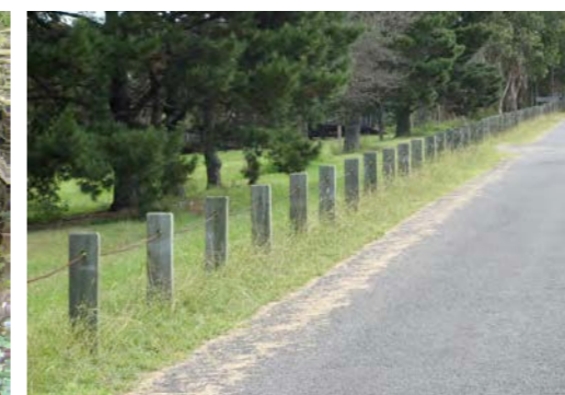
Post and cable barrier (Source: EP NSW)
