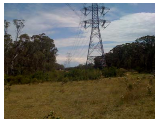
Site Image: Transmission lines (Source: EP NSW)
