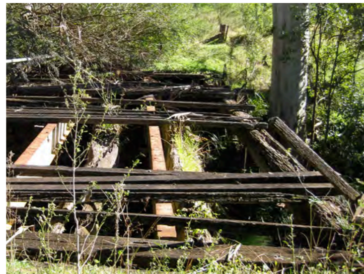
Upgrade bridge link across South Creek maintaining section of bridge as relic fabric (Source: EP NSW)
