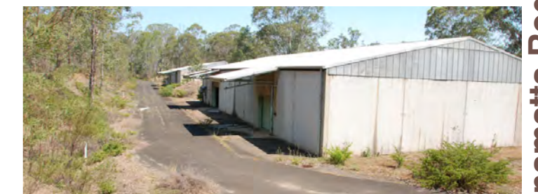
Reuse buildings 3 & 4 - multi-function space - potential usage • Shaded Parking • School camping/ education • Bike storage/ rentals
