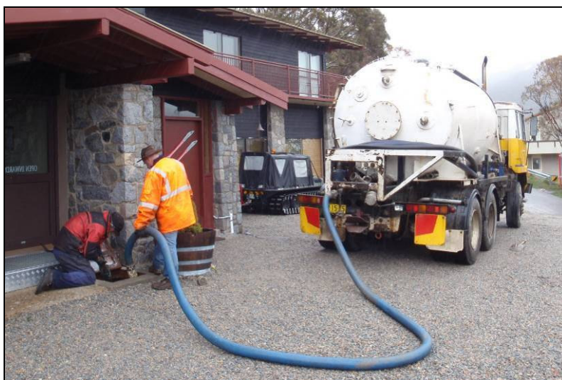
Figure 8 - Grease arrestor pump-out at Guthega (photo Tom Pinzone/OEH)
