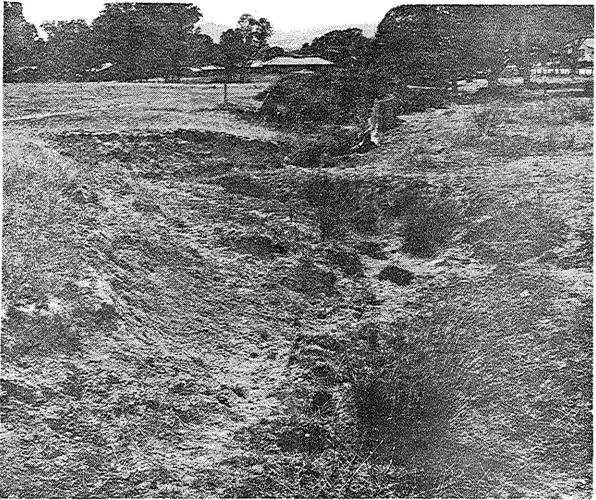
Figure 4. Incised channel of a fourth order stream. This land is sub-class D-2 and will require shaping as a drainage reserve.
