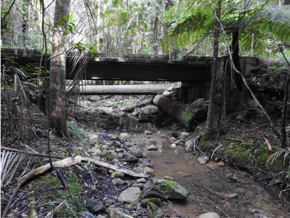
Photo 5 The road bridge over the western tributary above the Falls, probably the source of sediment affecting potential Giant Barred Frog breeding habitat
