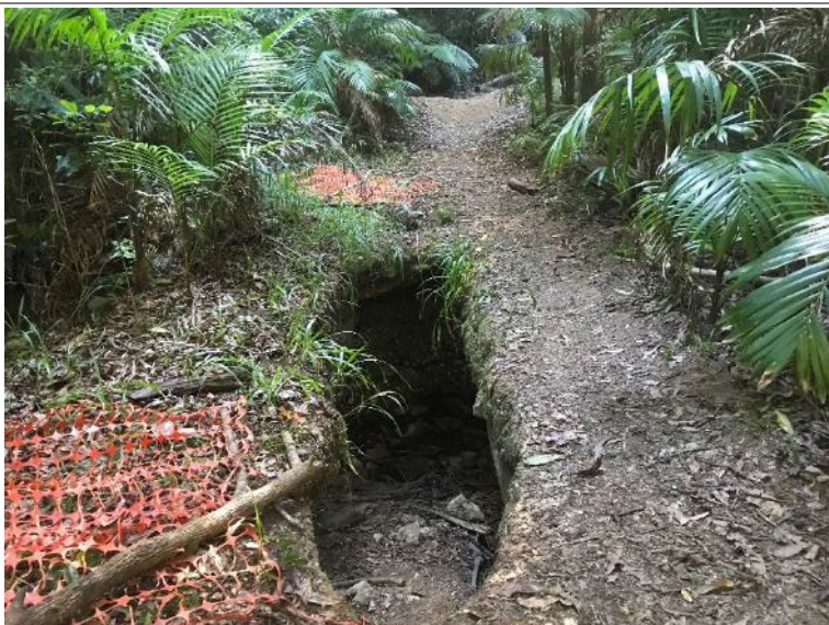
Plate 6. Bridge at Sand Ridge Road which will be repaired/replaced.
