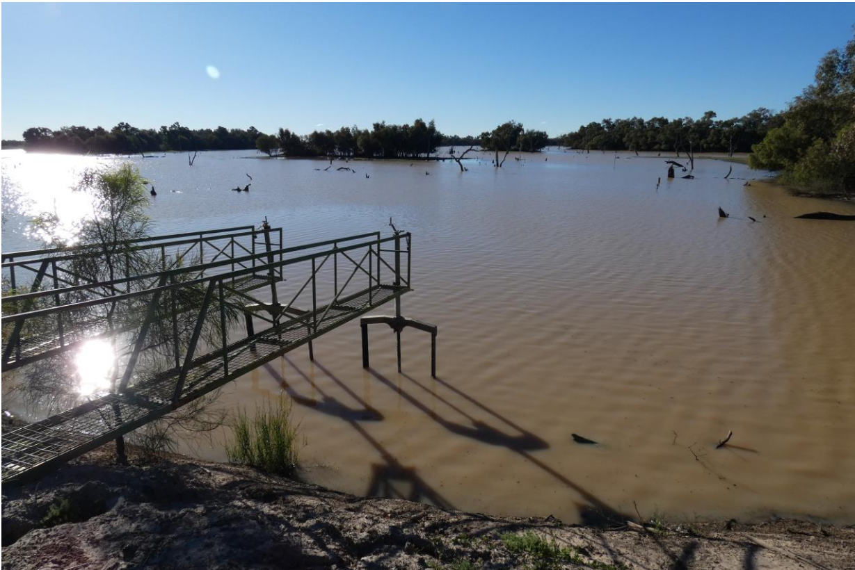
Figure 1-4: Existing conditions at Boera Dam. Platforms lead to the gates that can be opened to pass water through the dam and downstream into the Warrego River.
