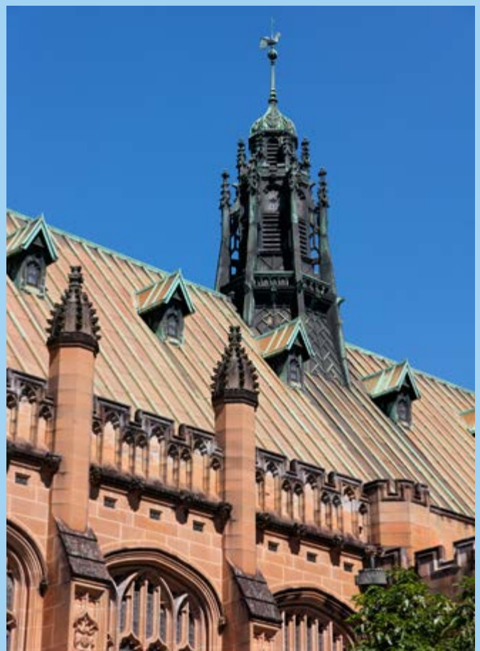
MacLaurin Hall viewed from the Quadrangle showing the copper clad central ventilating fleche with louvres at the upper levels on all sides (Photo: Steven Barry/Transport for NSW)
