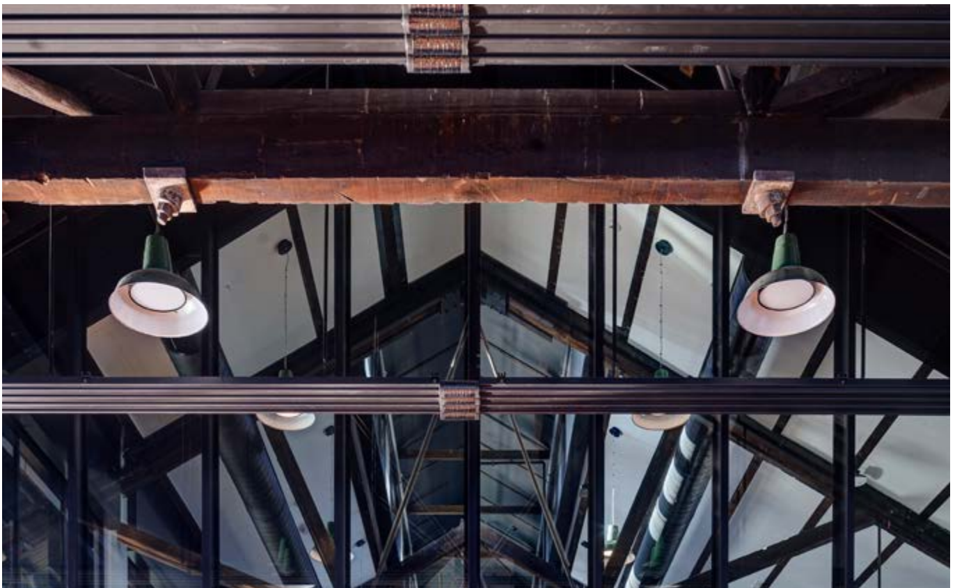
The redevelopment of the Walsh Bay Arts Precinct as a public arts and cultural hub in Sydney reused the existing enamelled pendant lights which were sensitively retrofitted with LED fixtures (Photo: Brett Boardman for TZG)
