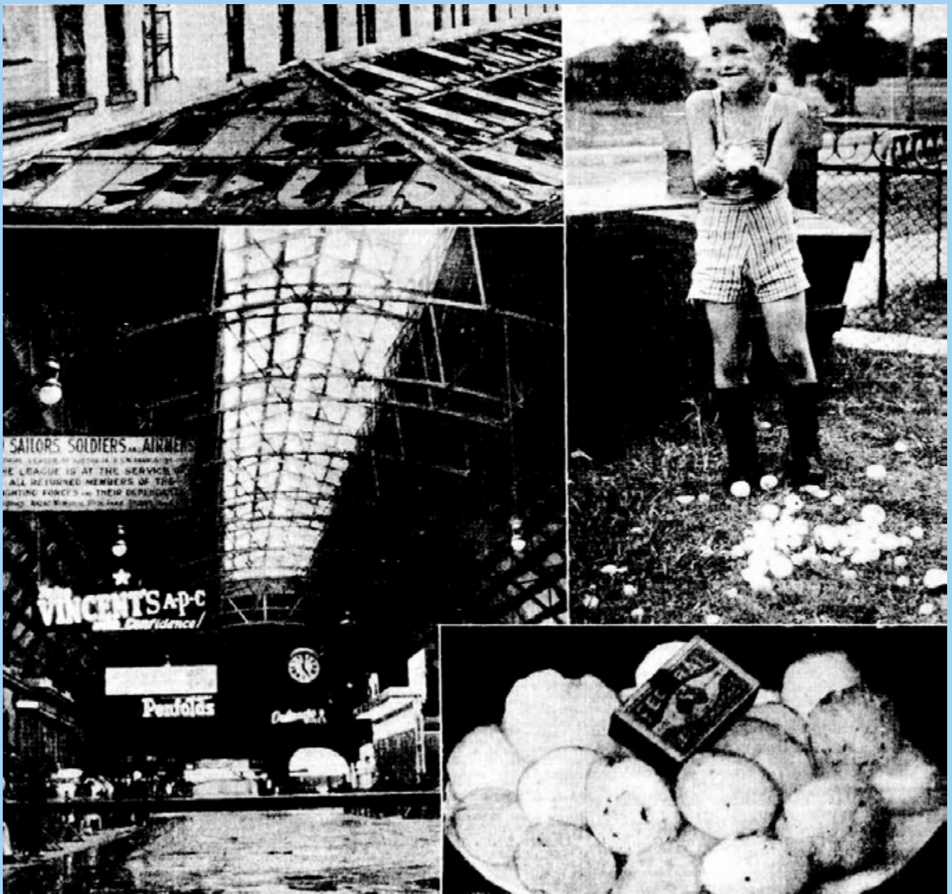
Image extract from January 1947 showing extensive damage to the Central Railway Station skylights which was the trigger for extensive replacement in less transparent or opaque materials (Photos: Sydney Morning Herald )
