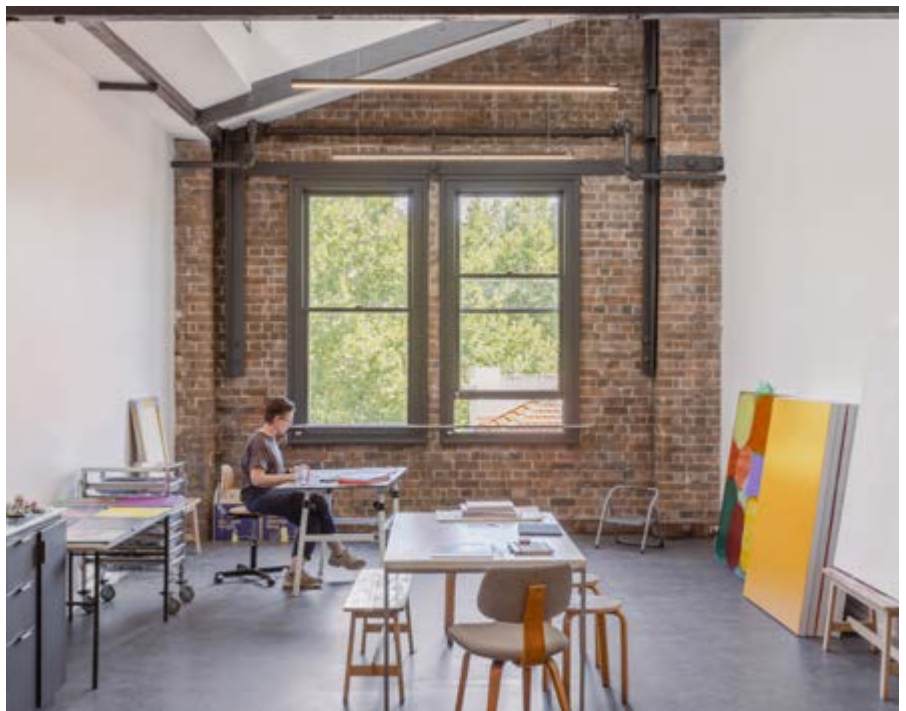
Typical timber sash window in the artist studios of The Gunner. Refurbishment works focussed on operability and addition of UV and security film to improve the environmental performance (Photo: Katherine Lu for DunnHillam)
