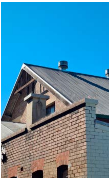
Coronation Hall, Newtown showing traditional roof cowls to the ridge connected to internal ceiling registers (Photo: Steven Barry/Transport for NSW)
