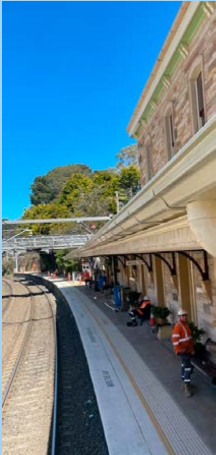
Completed image of the reinstated ogee eaves gutter (Photo: Transport for NSW)
