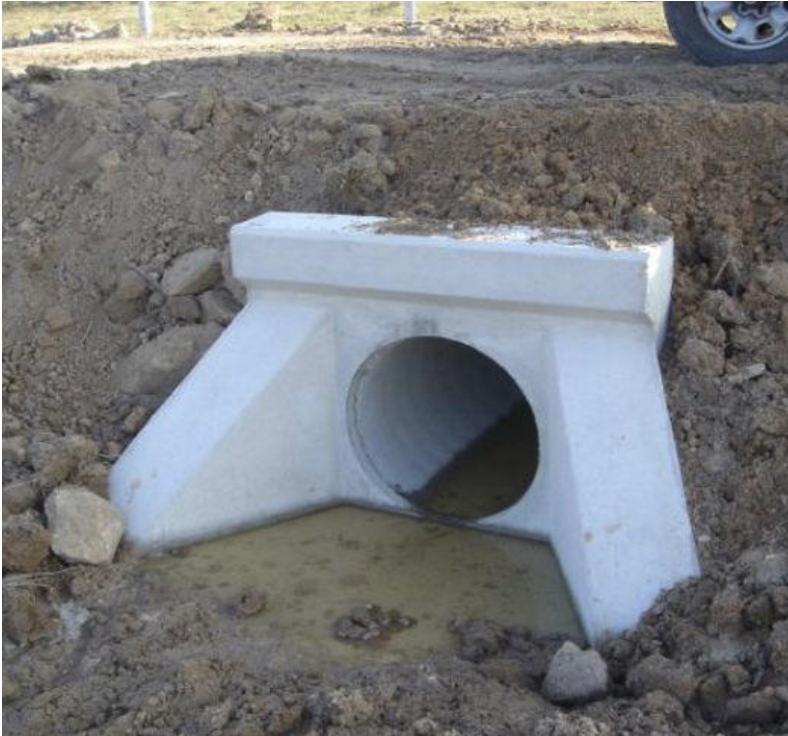
Figure 14: Example of a culvert and head wall that will be installed under the fence in areas where water is likely to flow
