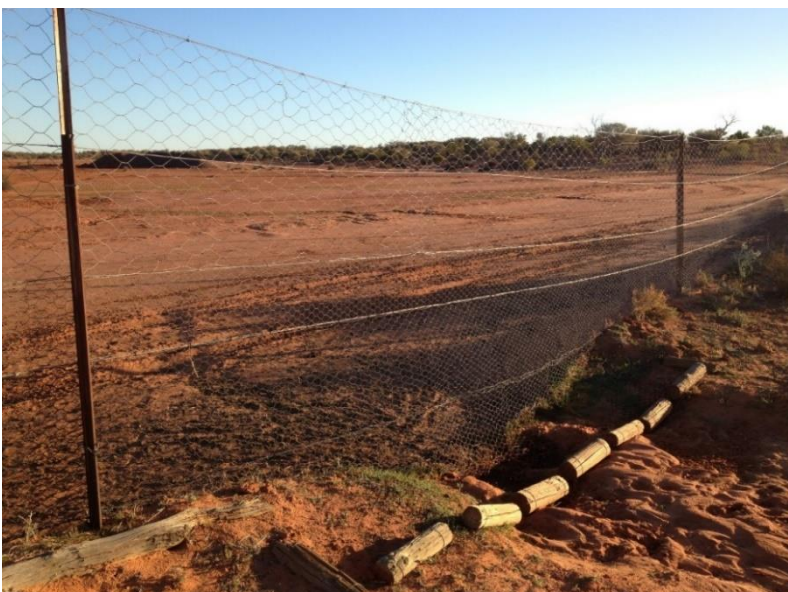
Figure 15: Example of a floating flood gate installed on the Dog Fence in areas where minor water courses intersect the fence line
