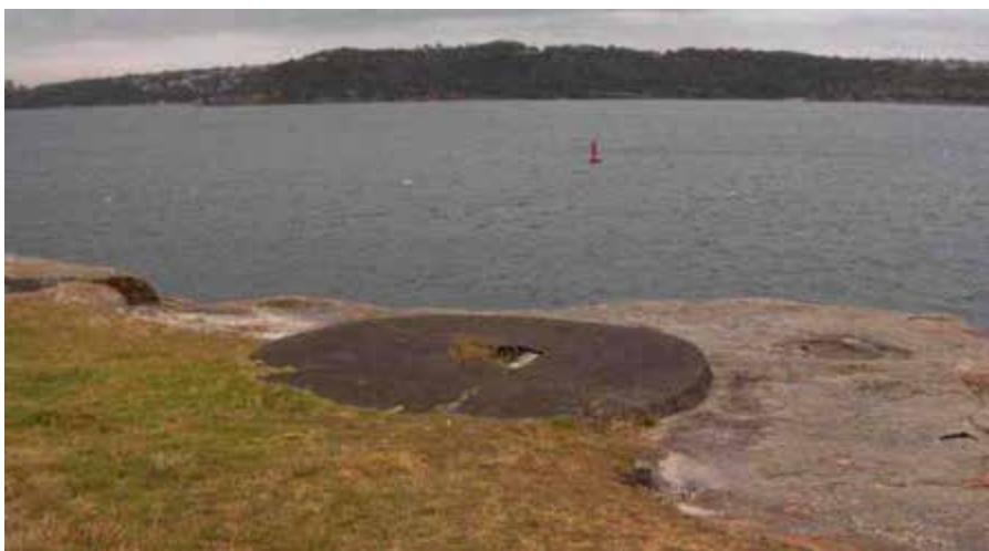
Figure 3.14. The concrete base of the flagstaff, looking south west over the harbour. October 2006
