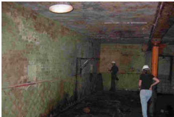
Figure 3.21. Interior of the Engine Room [1.3B] visited in 2006. Source: DECC 2006.
