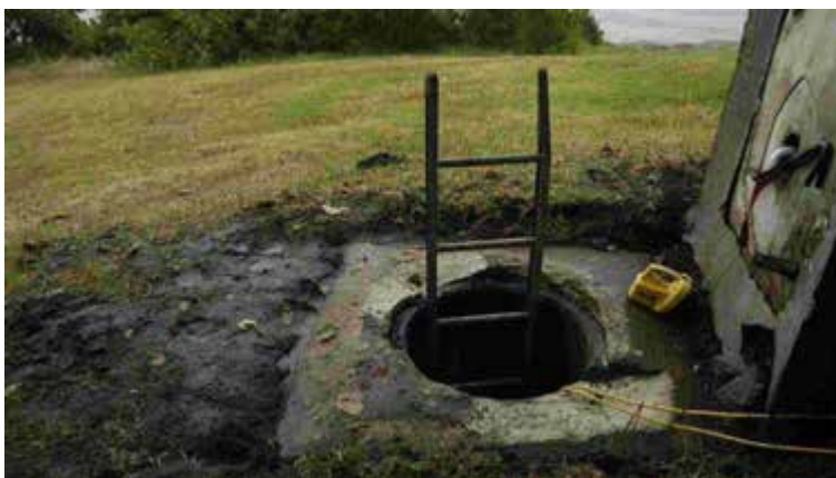
Figure 3.54. The current access to the Submarine Miners Firing Station opened for inspection in November 2006. Source: Paul Davies Pty Ltd November 2006
