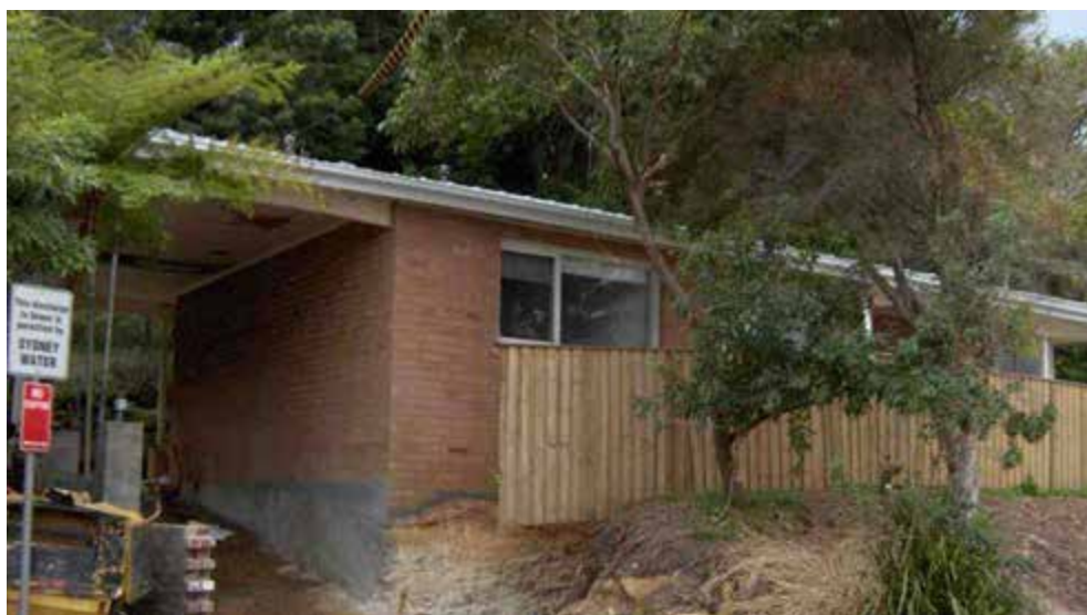
Figure 3.37. 33 Cliff Street during road and stormwater construction works undertaken by Woollahra Council. October 2006.
