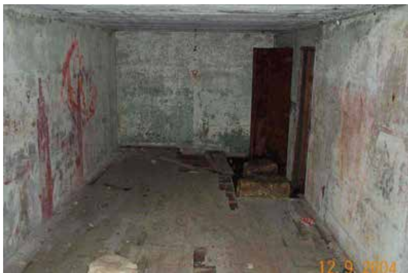
Figure 3.18. View of the interior of the Duty Room formed out of 1870s passage in 1939 showing the reinforced concrete ceiling, rendered walls and timber floor boards. Source: DECC 2004.
