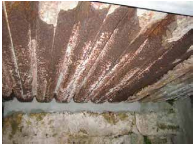
View of the rusted original Barlow rails supporting the concrete slab.
