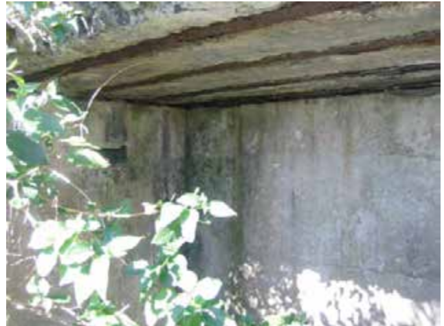
View of Item 2.8, between Camp Cove & Lady Bay Beach, remains of the 1890s searchlight observation station. The structure is partly collapsed. The roof slab is supported by rusted rail tracks. Further corrosion could lead to collapse.
