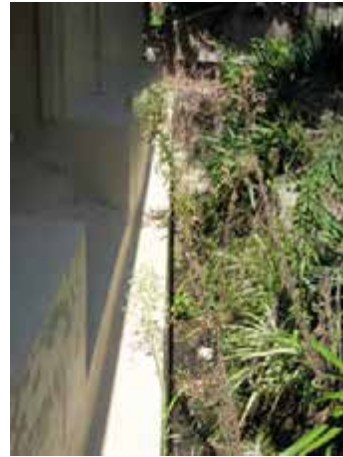
View of the rear addition, west portion, showing ground drain adjacent to building with plants encroaching.
