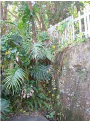
The drain is blocked by vegetation.
