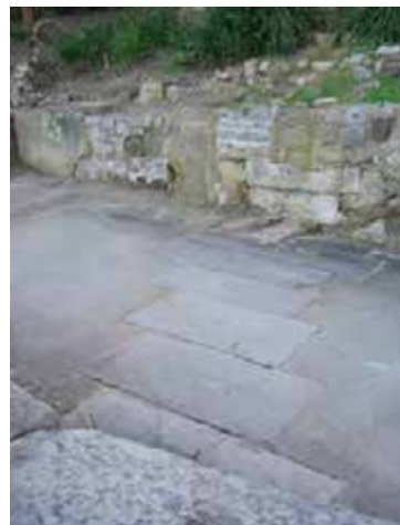
View of the pathway above Gun Pit with stone blocks that may indicate a drain under path.
