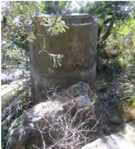
View of Item 2.3, North of Lady Bay Beach, the water tank is precariously balanced above partly collapsed structure.
