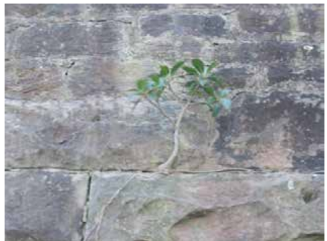
View of the rifle wall with a young fig tree growing in a mortar joint.
