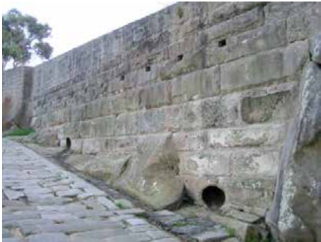
View of the rifle wall above Cobblestone Road. Noted two drains that should be inspected for blockages from above.
