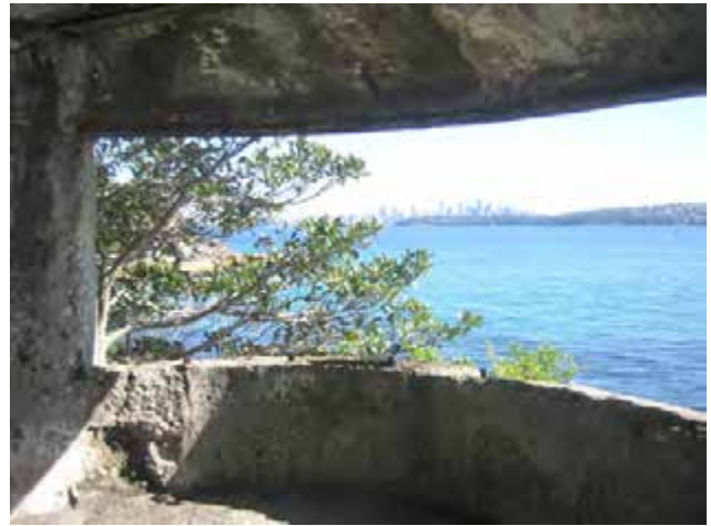
View of the opening to the harbour, looking west. The steel members supporting the concrete above opening are badly rusted. The fig tree, to the left, is growing in the structure.
