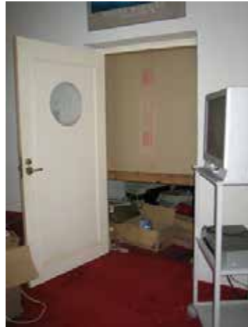
View of door in theatrette, egress route is blocked by construction of new room.
