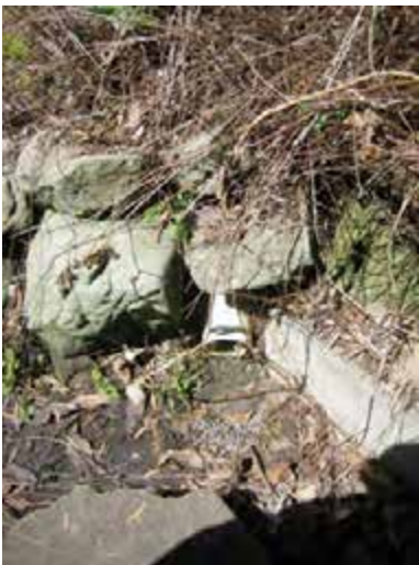
View of the stormwater pipe from adjacent property discharging into ditch with leaves.
