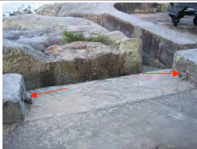
View of kerb to the access road with a missing stone block. Note the iron joggles projecting from the remaining stones. (arrowed)
