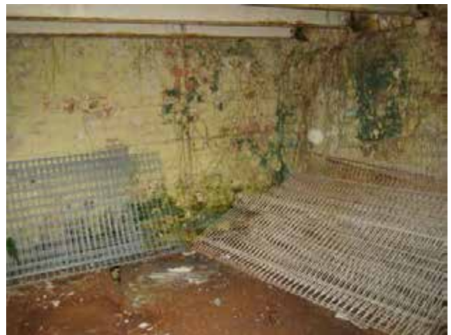
View of the building interior 4B.15, currently used for storage. In poor condition with deterioration of slab roof.
