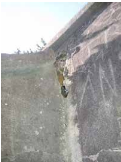
Detail of main entrance to underground structures. A large structural crack has opened up between the side and end walls. There has been movement in the structure.
