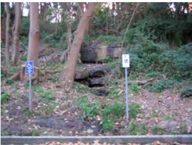
Water continually flows over this rock at the public parking area and may indicate a leaking pipe or similar above.
