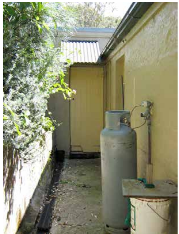
View of gas bottle, note area is only accessible through the building.
