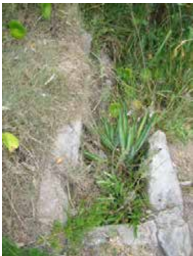
View of one drain, along the track above right, completely blocked by vegetation.
