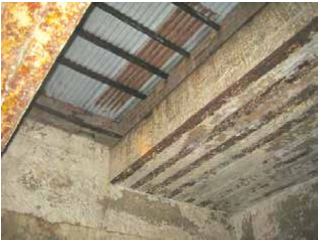
View of the skylight and roof. Note brickwork above original skylight walls. The slab to the right is supported by rail tracks which are visible.
