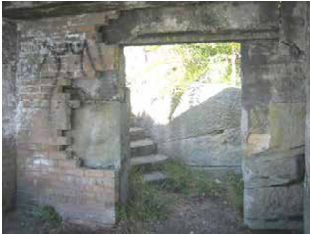
View of the entry from above. The lintel over doorway is rusted. Note the brick lining has been partly removed.
