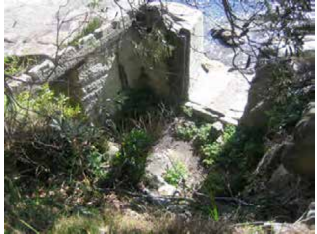
View of Item 2.3, North of Lady Bay Beach, the concrete roof has collapsed.
