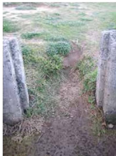
View looking out from Range Finder (DRF) showing water has been channelled into the structure.
