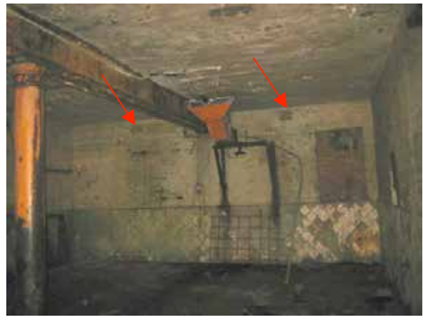
The north wall of the Engine Room showing the original white tiled dado, later painted green. Note the two vents (arrowed). At the right side of the beam are remains of machinery and ducts and at the right end of the wall a window that was bricked up.
