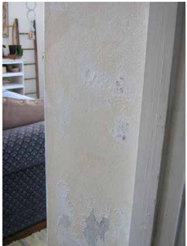
View of the salt damp in doorway.
