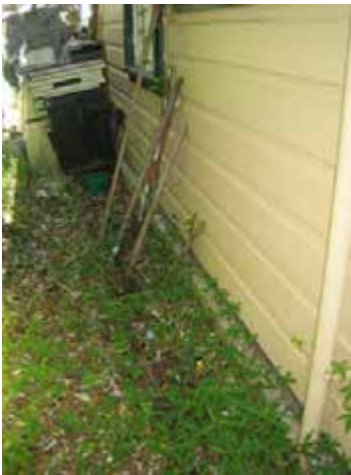
View of the building rear where drainage is blocked.
