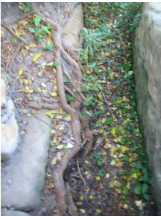
View of Gun Emplacement drain with roots blocking it.
