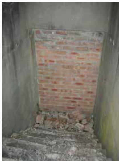
Exterior of door to Staff Room bricked up on exterior.
