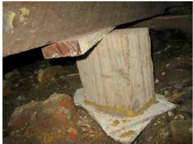
View of inappropriate footings with stumps glued over fibre cement sheets laid in bare ground and wedge at top.
