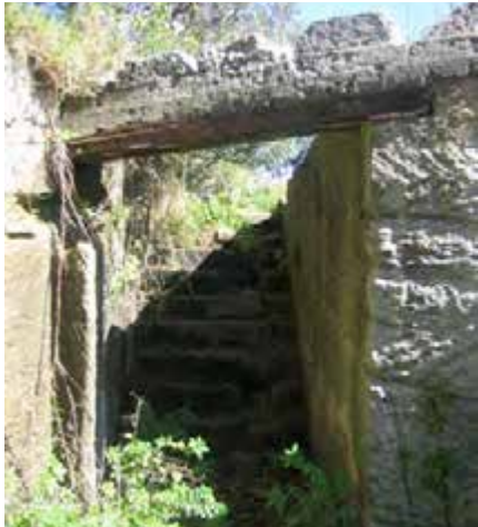
View of the access steps to structure showing the partly collapsed lintel that is unsupported on the left and is dangerous.
