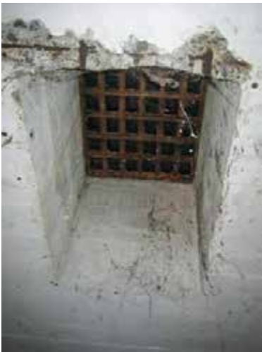
View of vent to exterior in the passage west of Shell Store. Iron grill over remains. Note concrete deterioration.
