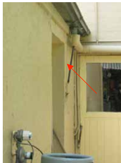
View of the rear plumbing to divert water from rear of building. Noted pipe is propped (arrowed).
