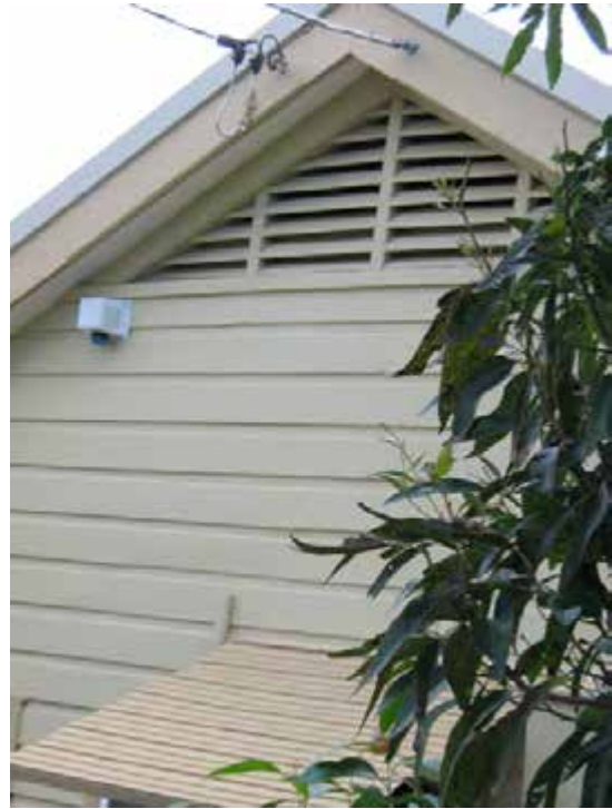
View of southern west front elevation, showing detail of ventilation louvres in the gable. Note modern services. There is a chamfered detail on the fascia indicating the location of the external louvres the same as those remaining at Gap Bluff Cottage.
