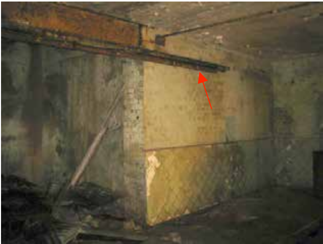
The east wall of the Engine Room to the right of the opening to the lightwell. The right sliding door track is arrowed.
