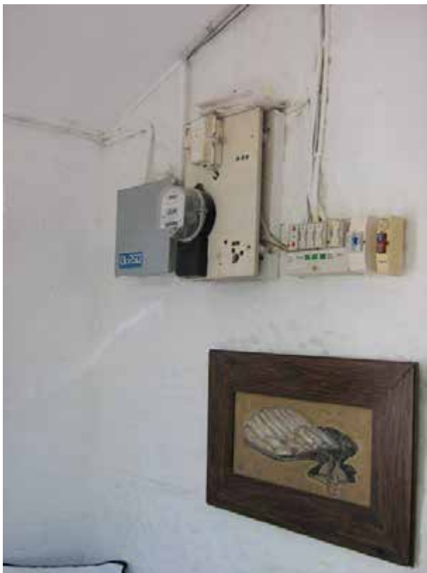
View of building services, power board and electrical services.
