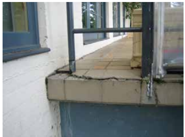
View of the modern verandah, front elevation (west), damaged rusting steel.
