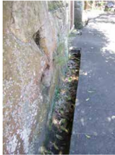
View of the drain at the cliff's base. Note that there are leaves inside the ditch and the drain is bridged at the former WC's.
