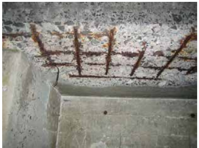
View of "concrete cancer" to a ceiling in some of 1930s sections of the structure.
