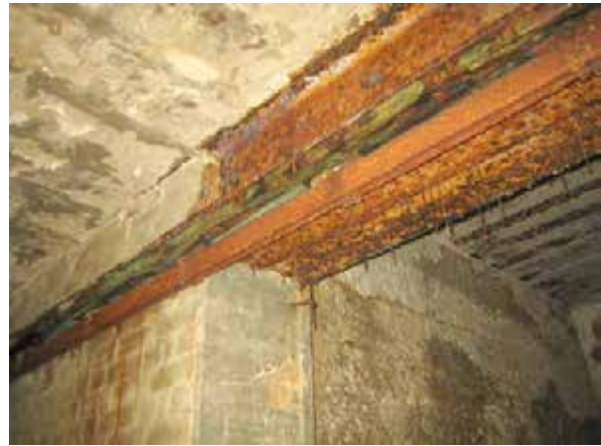
View of the steel beam over opening to the lightwell. The sliding door track crosses in front of the beam.
