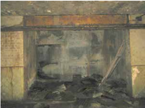
View of the opening to the lightwell with the passage, possibly connecting to the Staff Room, located the left side of the lightwell. Noted debris on the floor, mainly timber and cgi sheets.
