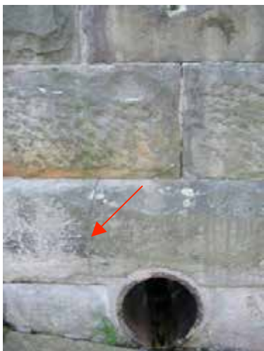
View of the rifle wall showing crack in the stone indicating some movement of the wall.
