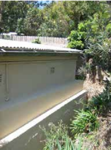
Stepped configuration of the wall makes it vulnerable to water entry.
