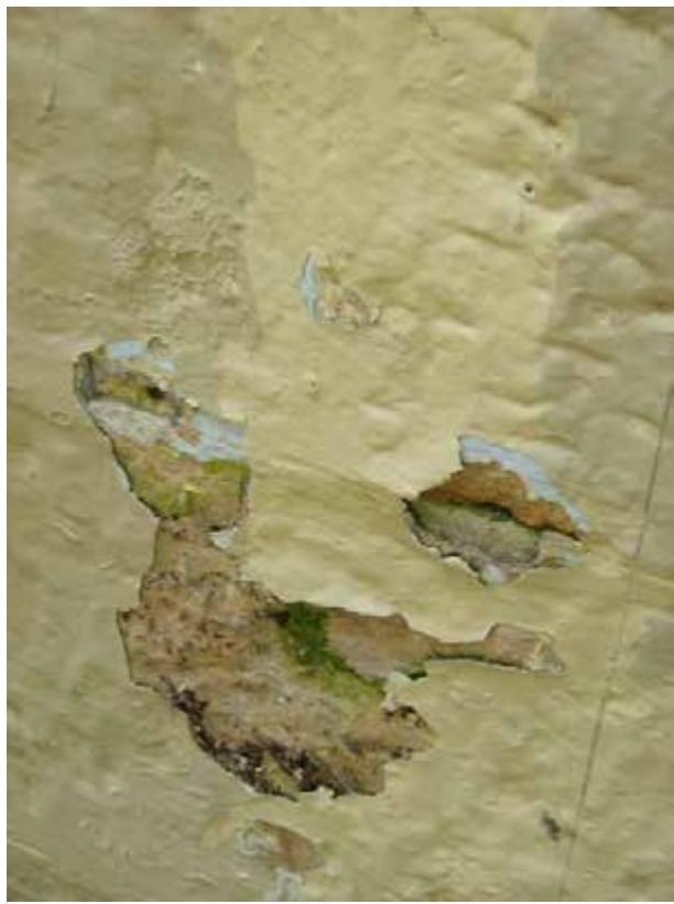
View of rear wall with damp and mould behind impervious paint.
