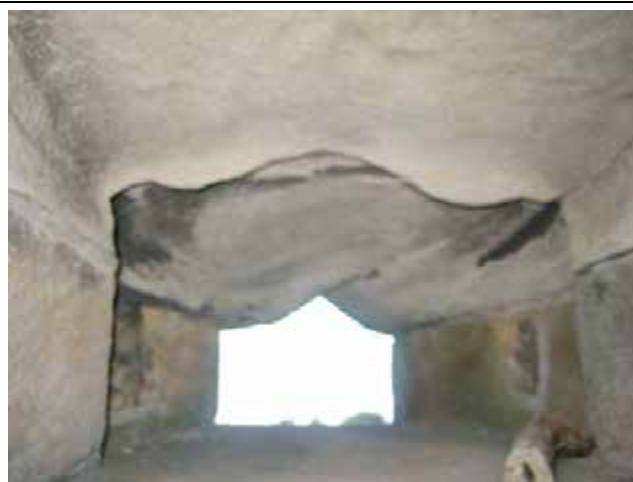
View of firing window [loop hole], showing detail of eroded stone.
