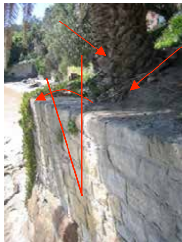
View of portion of the Lady Bay Beach retaining walls. Note the palm tree affecting the structural stability of the wall.
