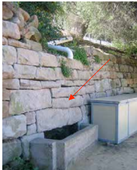
View of driveway retaining wall, at end of Camp Cove beach. Note stormwater pipe and that the stone lintel has a large crack.
