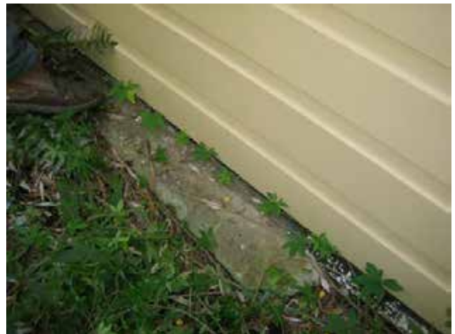
View of a section of earlier stone footing at building rear wall.
