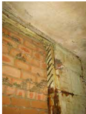
Former door opening in the south wall door showing frame with evidence of former louvres over door.
