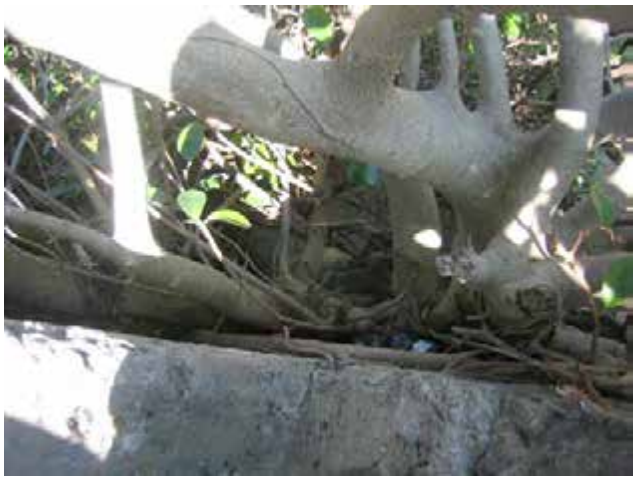
View looking down on the exterior at the fig tree has grown in the structure.
