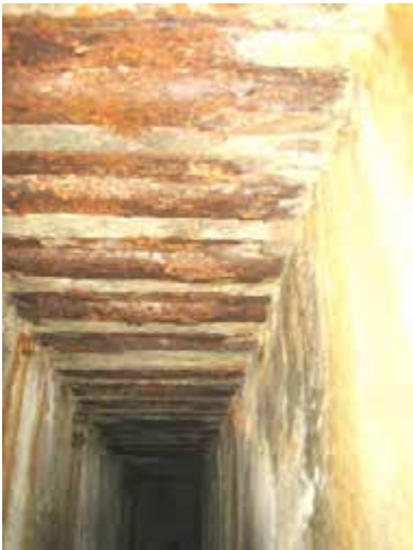
View of the ceiling of the passage showing rusted Barlow rails.
