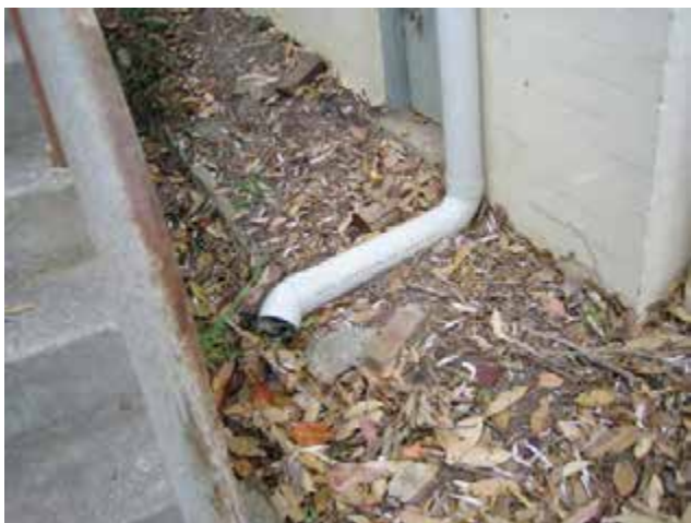
View of the downpipe discharging in open drain, blocked by leaves, at side wall.
