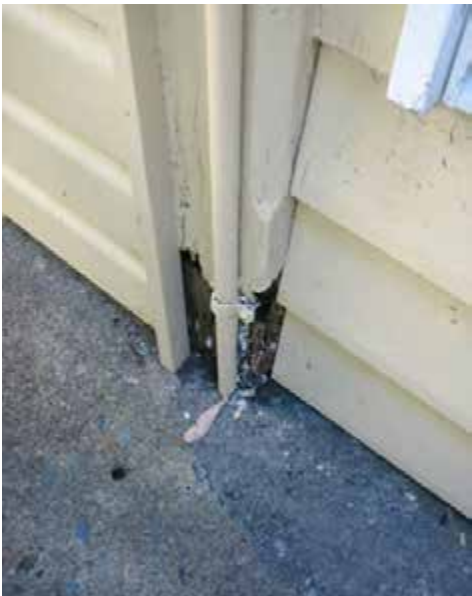
Exterior view showing rotted timber post base.
