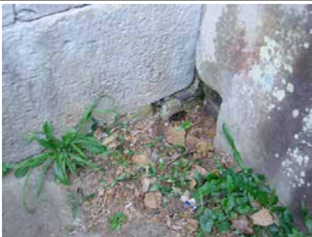
View of the stone drain, blocked with silt and leaves.
