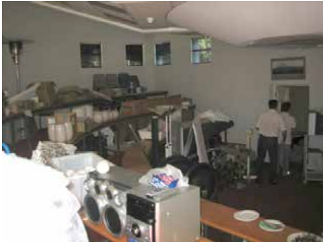
View of the lower floor theatrette interior, an addition to the building, used only for storage and suffering from damp.
