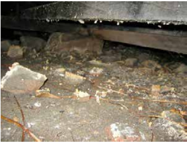
View of the underfloor space showing rocks used as footings. Note signs of damp and salts on rocks and minimal space under floor.
