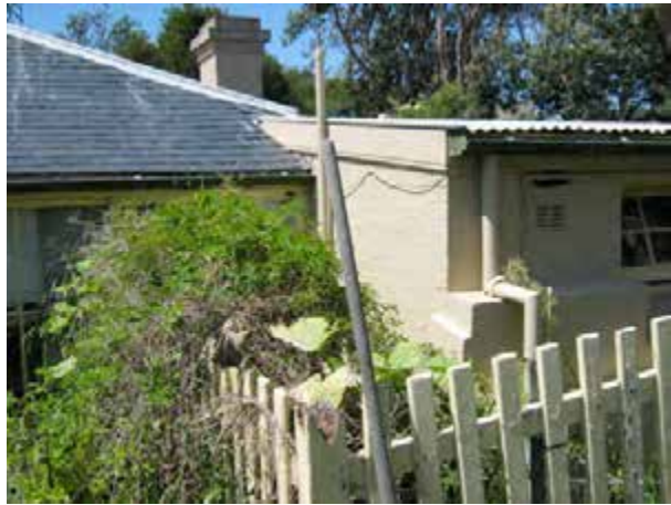
View of the rear addition, west portion, showing awkward roof junction and stepped downpipe.
