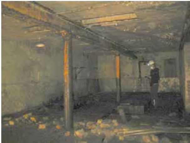
Looking north to Engine Room space. The room has two central columns under a beam running the full length of the space.
