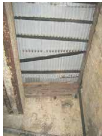
View of the current roof of the lightwell. Note that timber joists are collapsing. The area over is covered with soil. Is not known if there is any other structure above the "roof".
