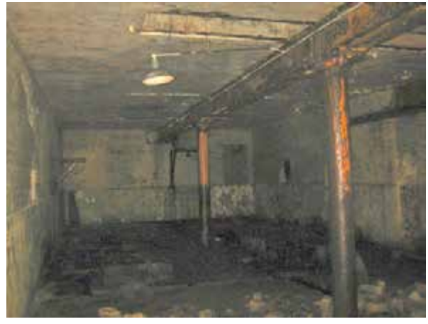
Looking south to Engine Room space. The space is rectangular the walls are brickwork with a tiled dado and have been painted.
