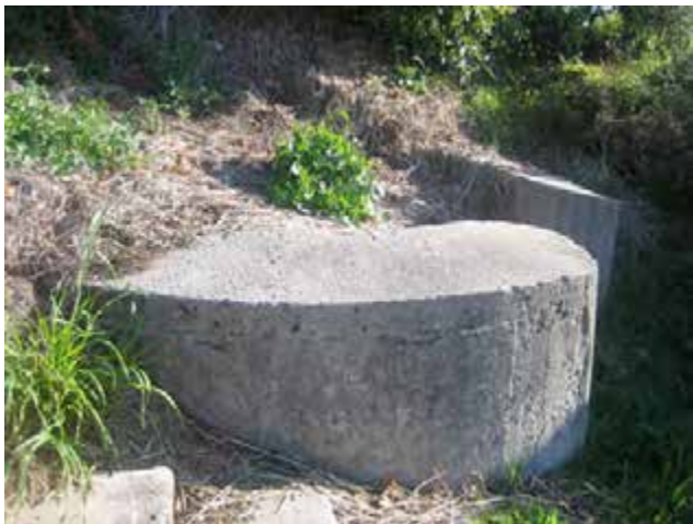
View of concrete structure, possibly part of an emplacement. Rubbish and vegetation accumulated over and in structure.
