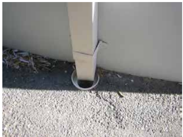
View of downpipe, outside building. As the room is damp drains such as this should be checked for blockages and correct function.
