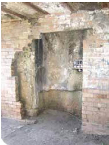
View of the Searchlight interior, north wall, showing that the structure is cut out of the rock and then lined with brick. Some of the bricks have been removed.
