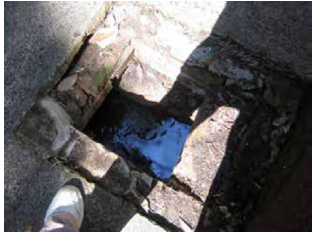
View of the drain / sump with slime and evidence of damp.
