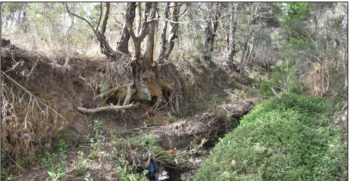
Figure 21 Active gully erosion in the central drainage plain, caused by urban stormwater run-off. Photo: Casey Murphy/OEH
