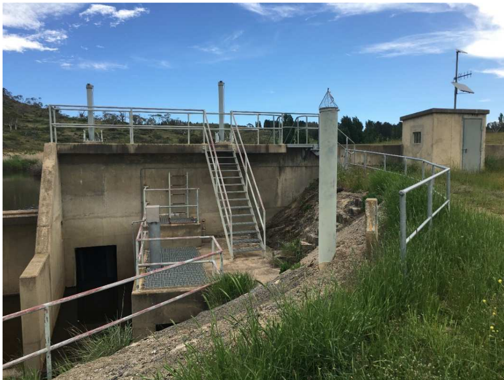
Figure 33: Mowamba Weir showing drain gate (dark rectangle), with the weir crest to the left
