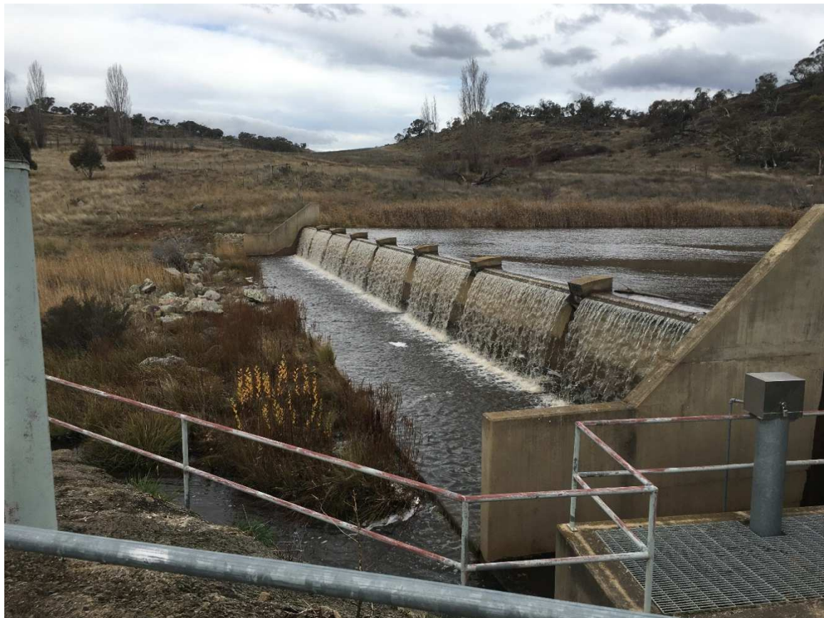
Figure 31: Mowamba Weir with an overtopping flow on 13 May 2021
