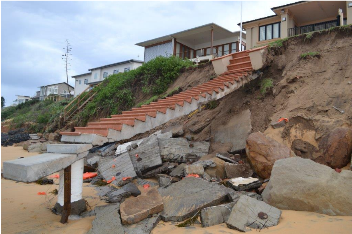
Figure 2 Erosion at Wamberal beach caused property damage and a public safety risk, June 2016 (Photo: D Hanslow/DPIE)
