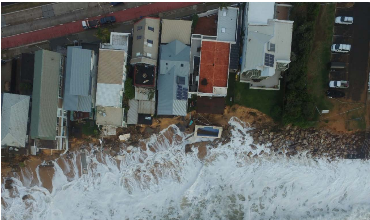
Figure 3 Extensive damage to private property and utilities resulting from erosion at Collaroy Beach following a severe coastal storm (Photo: UNSW Water Resources Laboratory)
