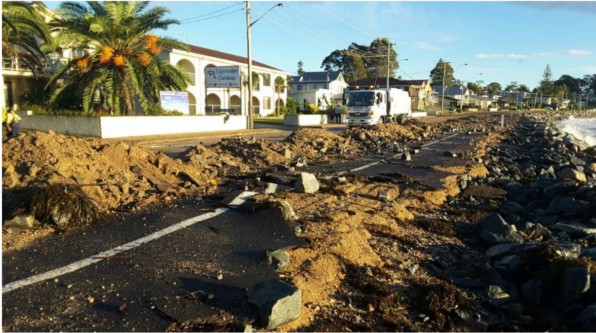
Figure 5 Damage caused by coastal inundation (Photo: G Armstrong/Eurobodalla Shire Council)
