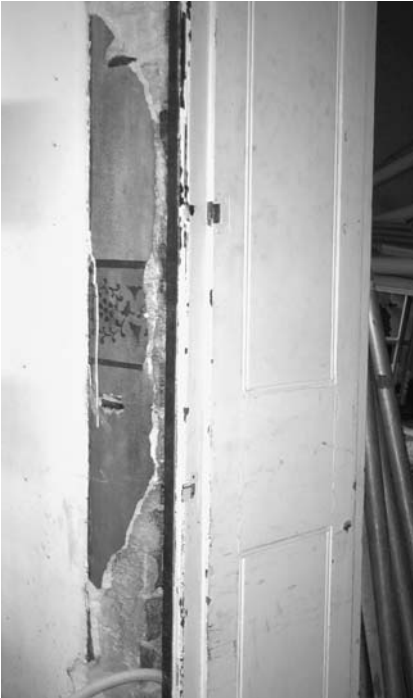
Removal of an architrave at the Chief Secretary's building in Sydney has revealed the earlier decorative paint scheme.
