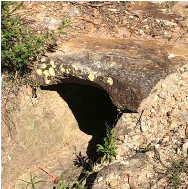
Figure 3.12: Stone culvert with curved lintel, Devines Hill. (Photo: Richard Mackay, Mackay Strategic Pty Ltd, 2018)
