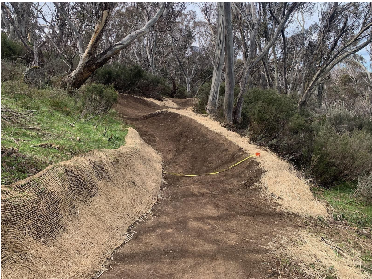
Figure 26 Recording monitoring points on a new gravity trail in the Thredbo Mountain Bike Park
