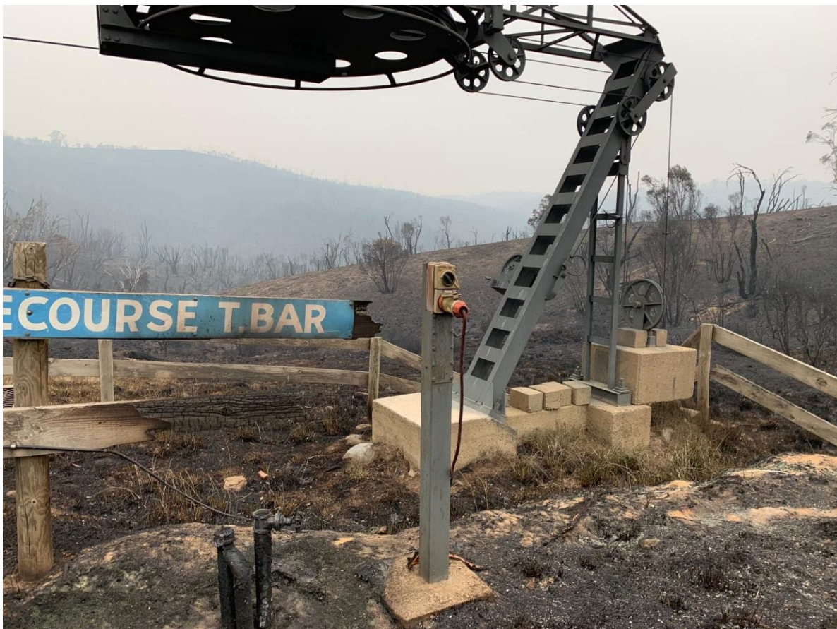
Figure 2 Damage to a Selwyn Snow Resort T-bar after the 2020 bushfires Photo: A Murdoch/Blyton Group
