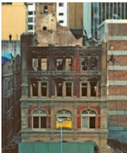
91 : The building damaged by fire in 1996.
