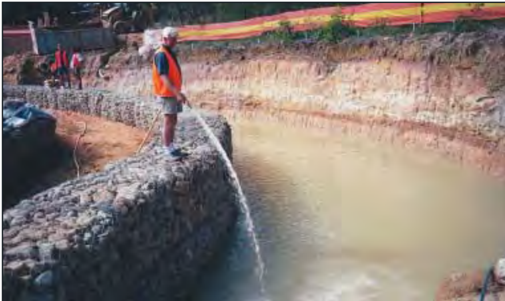
Figure E2. Poor gypsum application technique.
