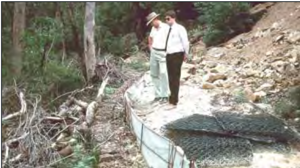
Figure 6.9 Sediment fence constructed below a fill batter – the sediment pollution is the result of a recent storm event
