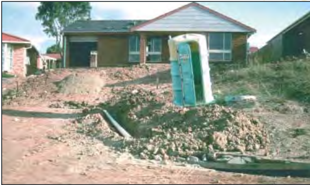
Figure 6.1 Sediment deposition below a housing construction site. As a result, the bitumen road and kerb and gutter are barely distinguishable – only a drop inlet is clearly visible
