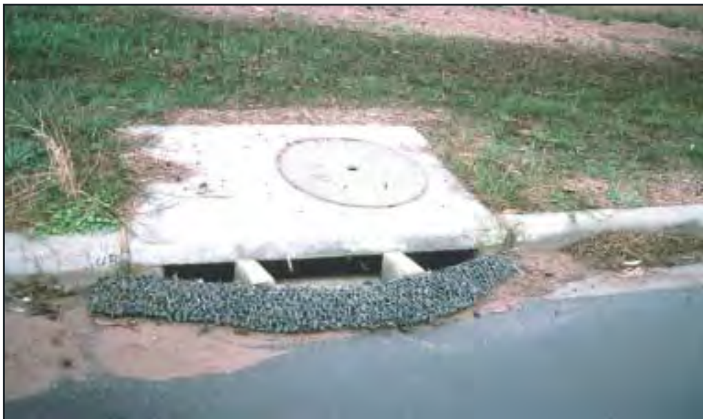
Figure 6.11 Filter roll at kerb-side sump
