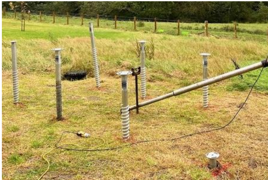
Example of foundation type 1 ground screw
