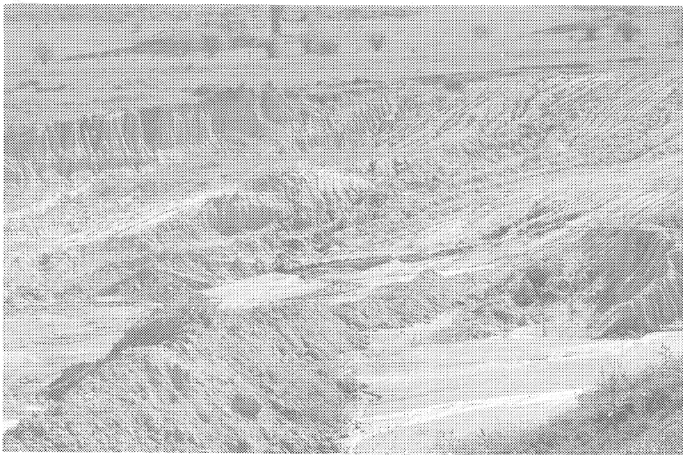
Many gravel pits are left in an eroding and unstable condition. They are contributing to the siltation of streams in the Designated Area.
