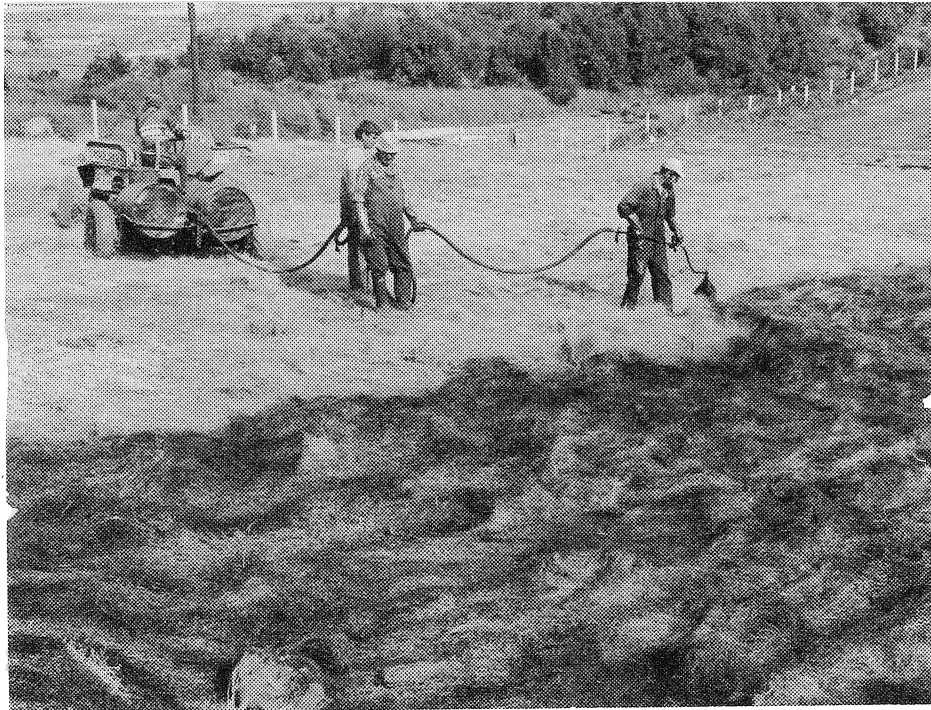
Revegetation of critical areas with hay mulch and bitumen is required on highly erodible soils.
