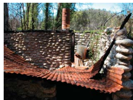
Figure 1.1 Dr Forbes' Hut, Geehi, badly damaged by bushfire in January 2003. Approximately a quarter of the hut and standing ruin hut resource was impacted by these disastrous fires.
