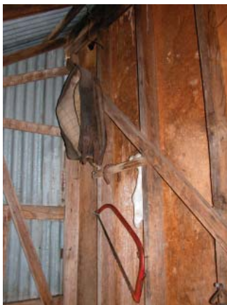
Figure 3.56 Timber stud frame clad with corrugated iron (Mawson's interior, 2004). Also showing caneite panels.
