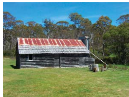
Figure 3.59 Roof of Tin Mine Barn combines timber shingles and short lengths of corrugated iron. 57
