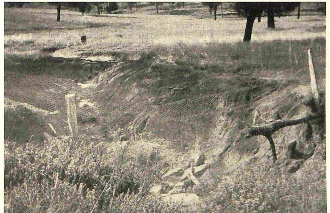
Fig. 3.—A gully on "Gilgai" prior to treatment. Discharge from the roadside was the cause.
