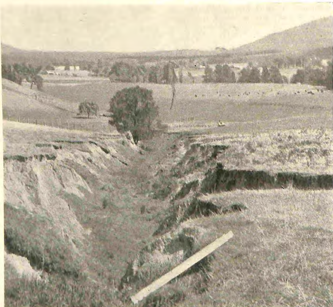
Fig. 3.—These gullies which formed in arable land are now stabilised by a change in land utilisation involving protective pasture cover.
