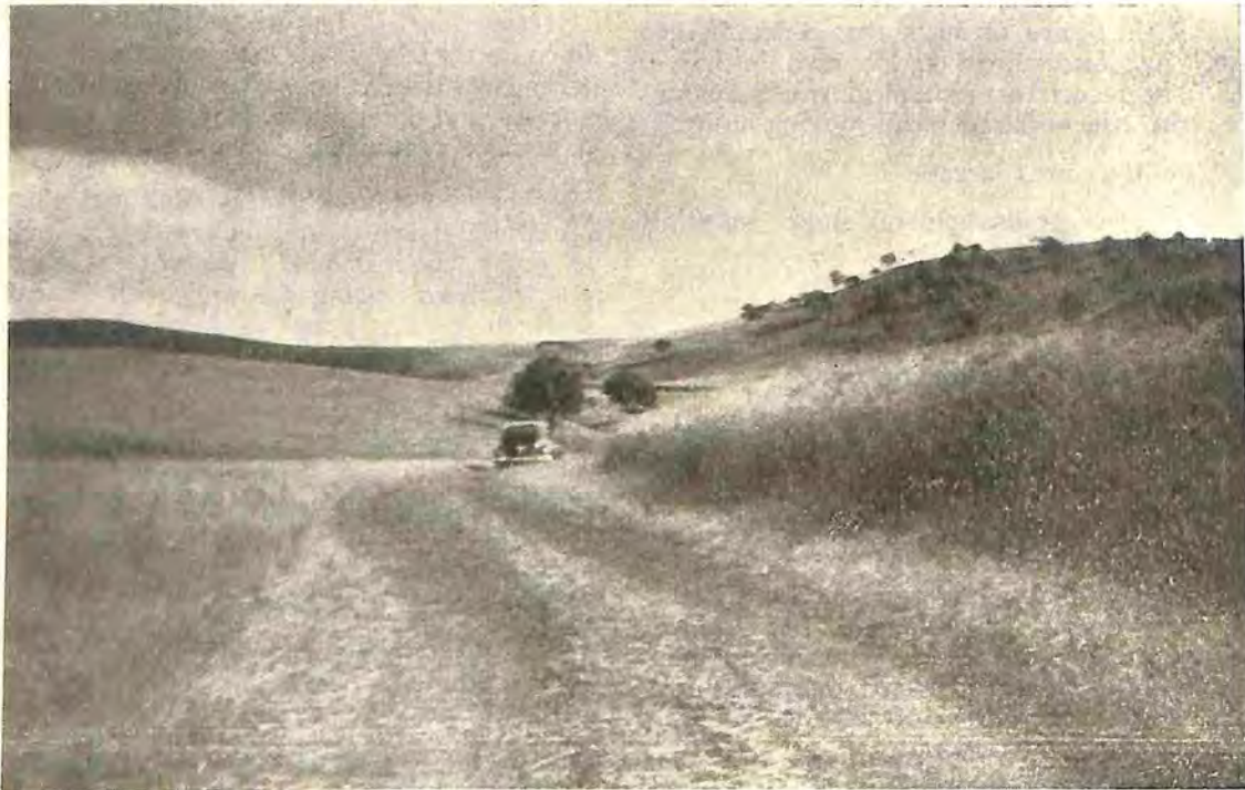
Fig. 1.—A contour track on Scone Research Station constructed immediately below a bank supporting a dense cover of Rhodes grass.
