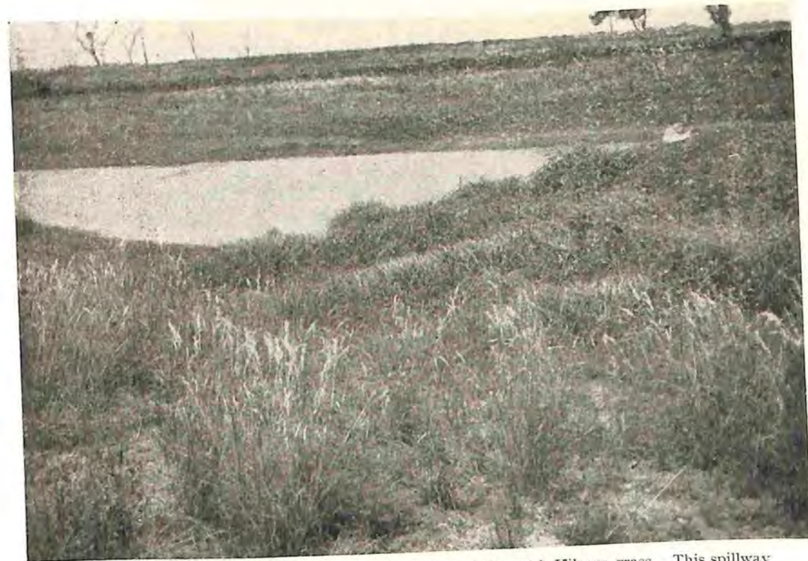
Fig. 1.—A farm dam spillway ten weeks after strip sodding with Kikuyu grass. This spillway has carried a twelve inch overflow for several hours safely.
