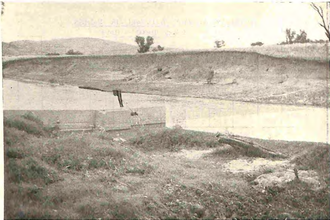
Fig. 2.—General view of the eroded river bank of the Namoi River adjacent to the Manilla weir.
