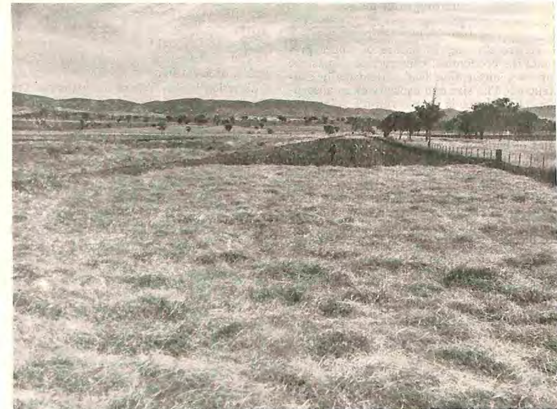
Fig. 3.—A view looking along a newly constructed waterway in the Tamworth area. Note straw mulch in foreground.
