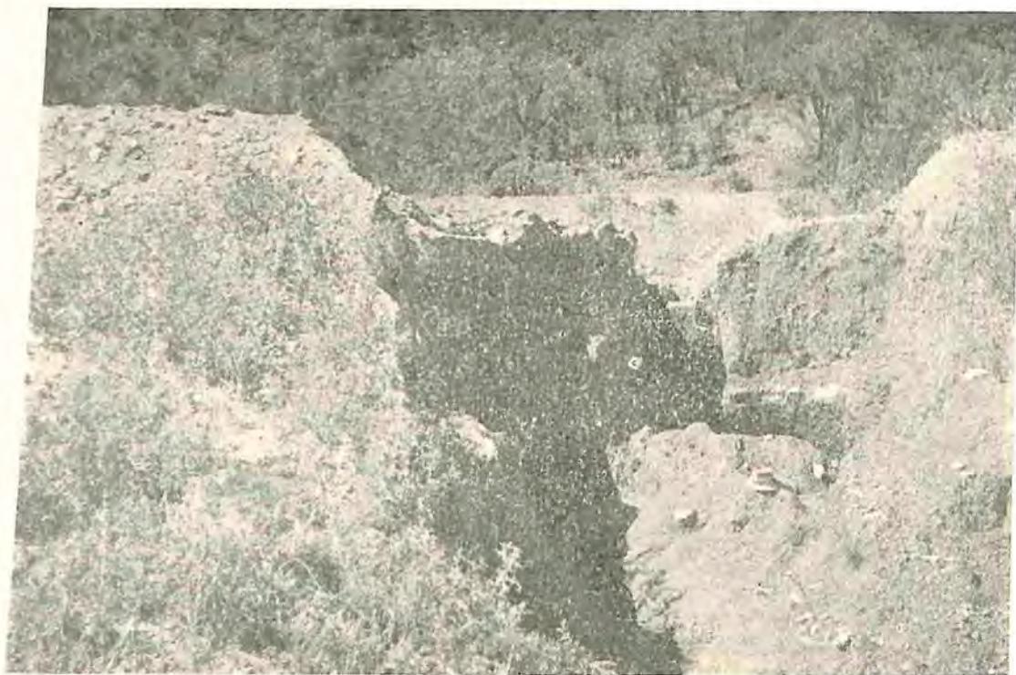
Fig. 5.—A badly-designed silt trap. Settling of the wall caused the water to flow over the top of the wall instead of through the outlet.
