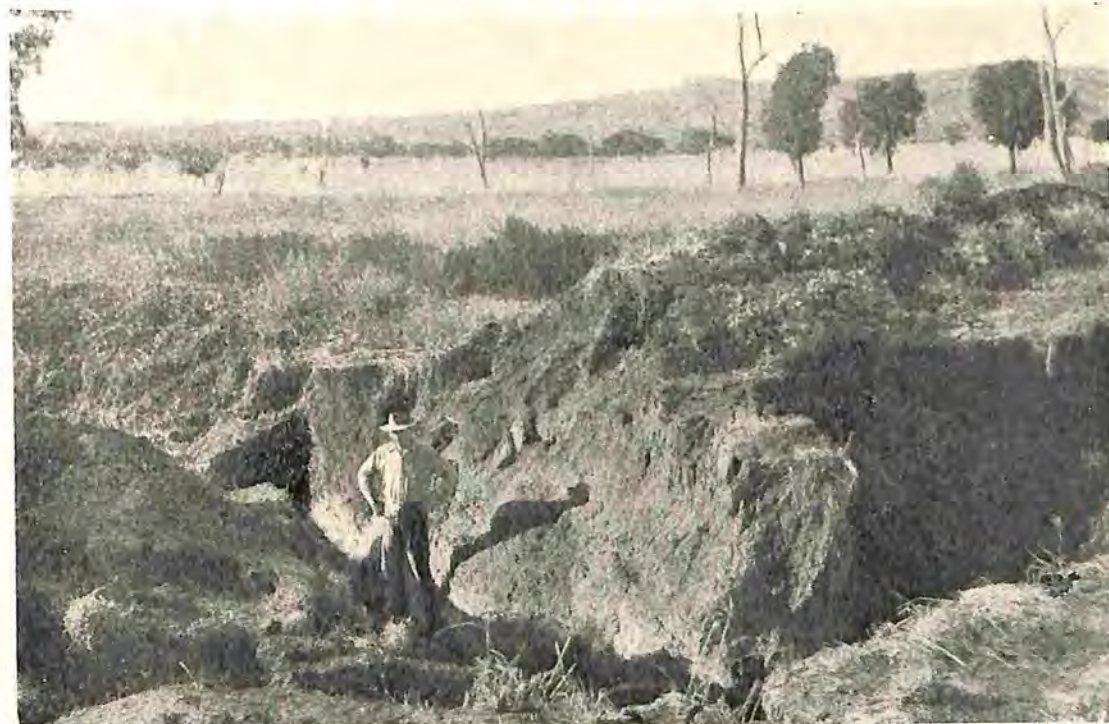
Fig. 4.—The damage to this absorption bank was caused by the water seeping through the bank, where it crossed a gully and eventually undermined it. This could have been prevented if the gully fill had been properly packed.
