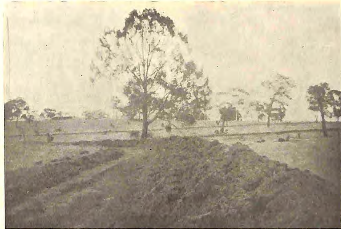
Fig. 4.—Bank construction on heavy black clay soils, using farm grader on ploughed strips.
