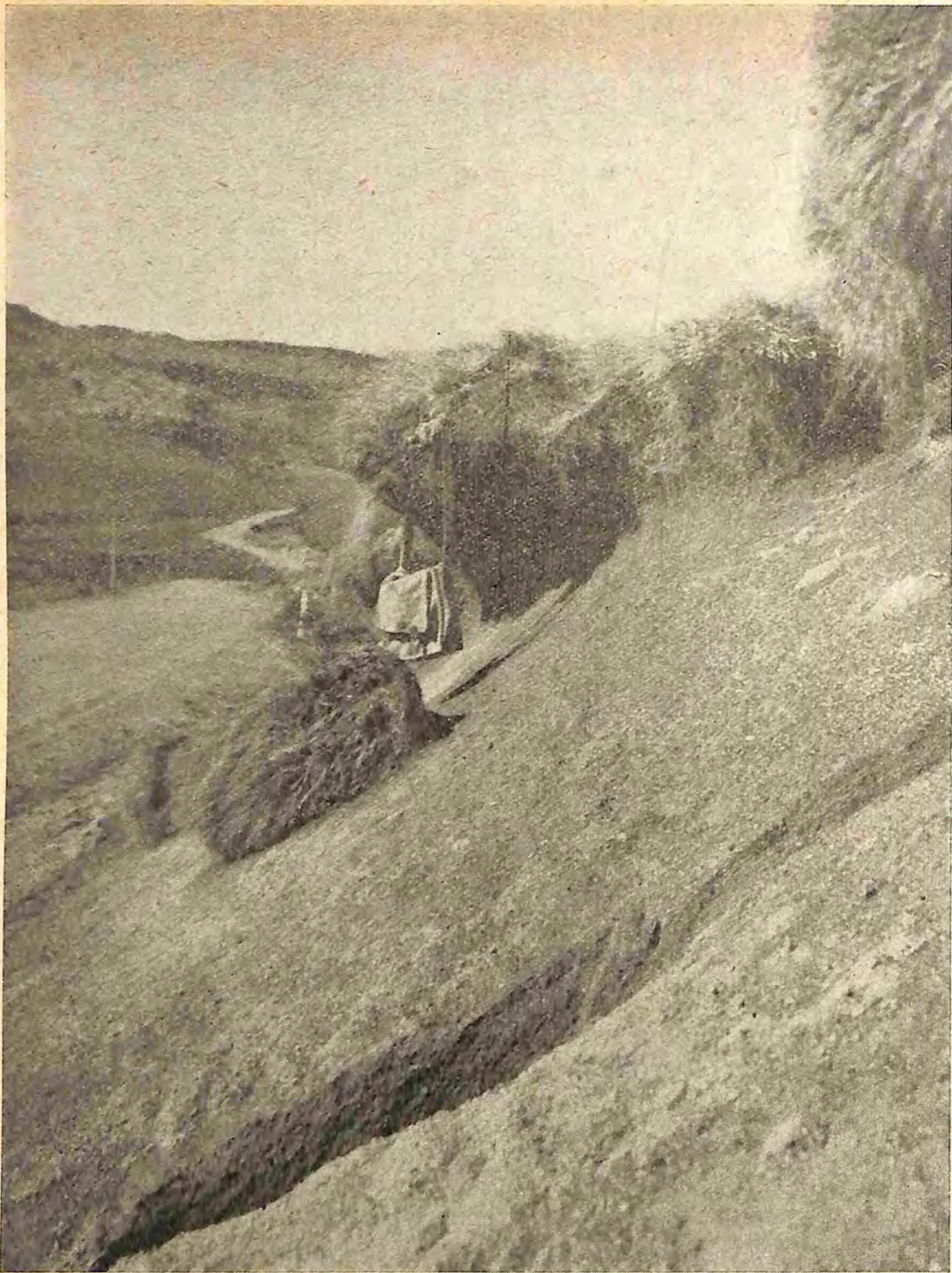
Fig. 8.—Recession of roadside cutting in sub-alpine tract, due to vigorous frost action followed by caving of the undermined surface soil.
