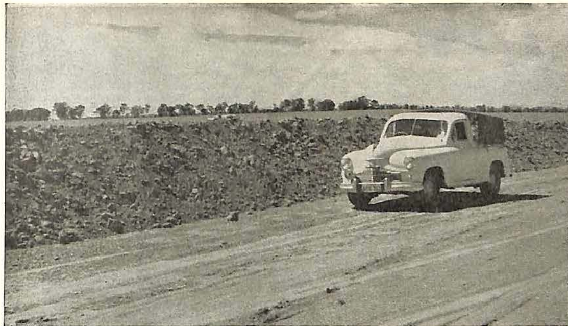
Fig. 3.—A massive absorption-diversion bank constructed by the Soil Conservation Service in the West Wyalong district.
