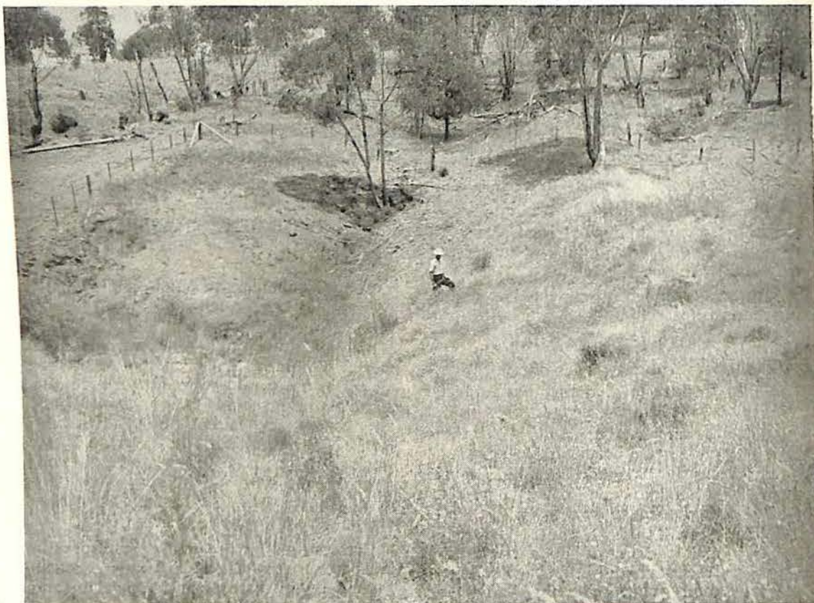
Fig. 2.—Back batter of dam wall completely stabilized with ungrazed Kikuyu grass. Note rilling on unplanted areas.
