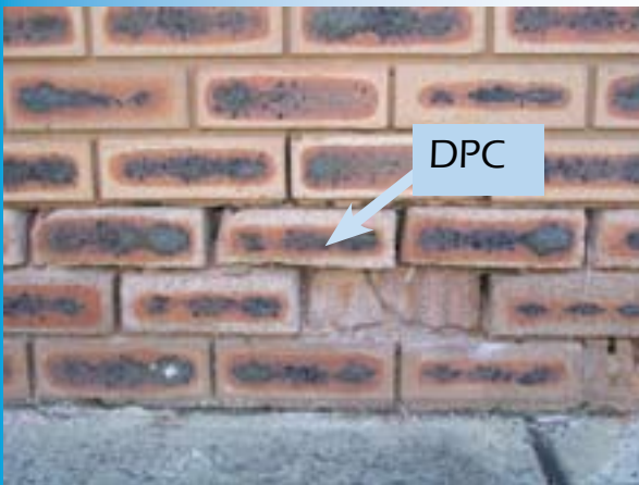
Salinity damage is minimised to the area below the damp proof course (DPC) in this building. Photo: Campbelltown Council
