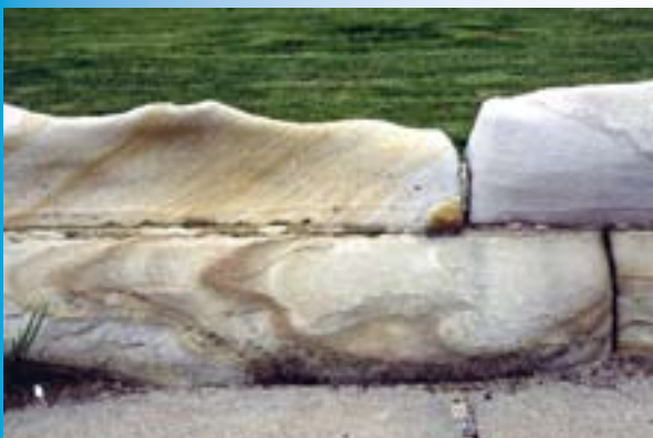
Salt action has damaged this sandstone wall in central NSW. Photo: NSW DPI
