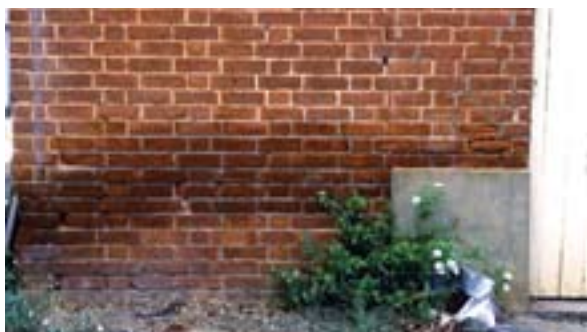
Tide mark on wall indicating the presence of water. This could be groundwater close to the surface or a leaking pipe. Photo: NSW DPI.
