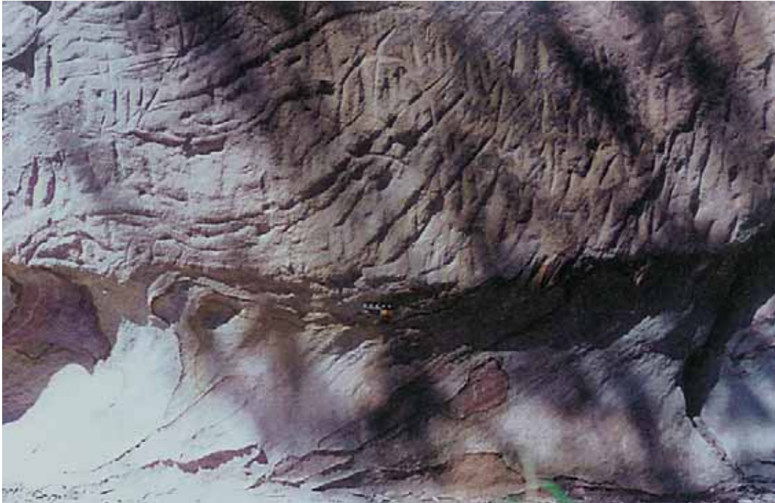
Plate 14: Salt weathering undercutting engravings at Pilliga Nature Reserve north of Coonabarrabran.
