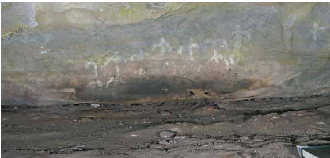
Plate 2: The same site after treatment for dry lichen. Note that it is difficult to completely remove dry lichen.
