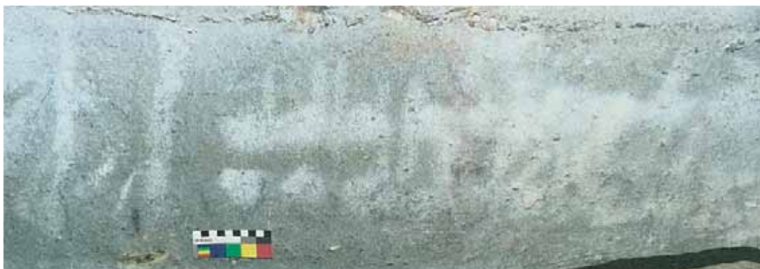
Plates 29 and 30: show the results of removing graffiti by dry brushing at Appletree in Wollemi National Park. Note that remnants of the charcoal graffiti remain but the visual impact of the graffiti is greatly reduced.
