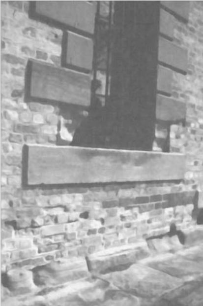
Rising damp in brick and stone masonry. Note how the worst decay is at the base of the window opening. This is where most evaporation takes place and hence most decay due to salt attack.
