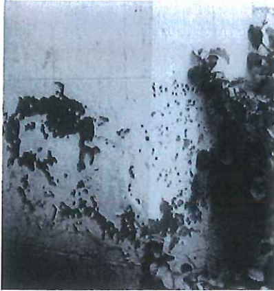
A modern paint coating, consisting of fine aggregate bound with resin, spalling less than two years after application to an 18th-century wall.
