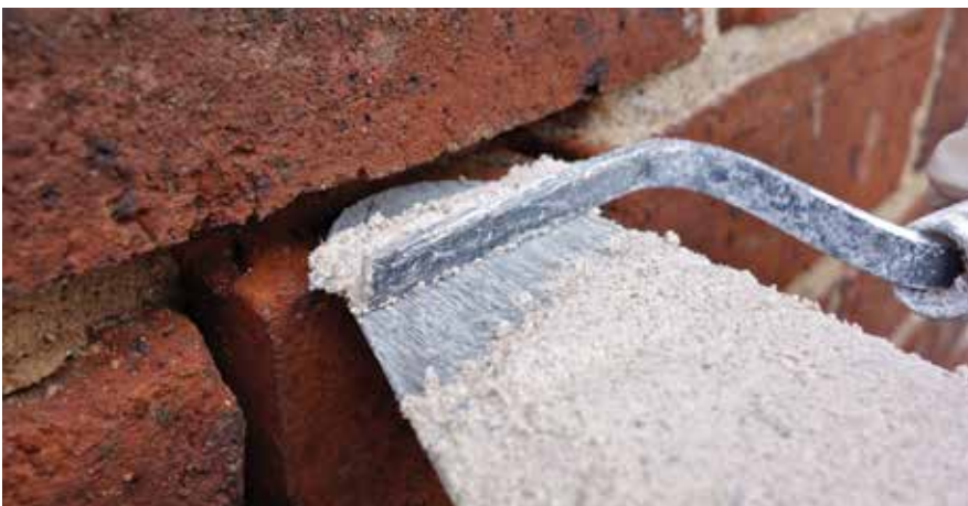
Figure 69: Using a trowel as a hawk. Speeding up delivery of mortar to a bed joint by using a gauging trowel as a hawk. Provided the underside of the trowel is kept clean, there need be no mortar stains on the face of the brickwork. A plastering trowel can be used in the same way.
