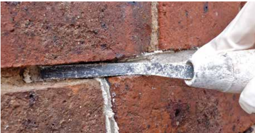
Figure 67: Filling a bed joint. An 8 mm trowel is used to place a small amount of mortar at the back of the raked-out joint; this is repeated until the joint is filled. The mortar is tightly compacted into the joint and also back into the last-filled section. This means working from right to left for a right-hander and left to right for a left-hander.
