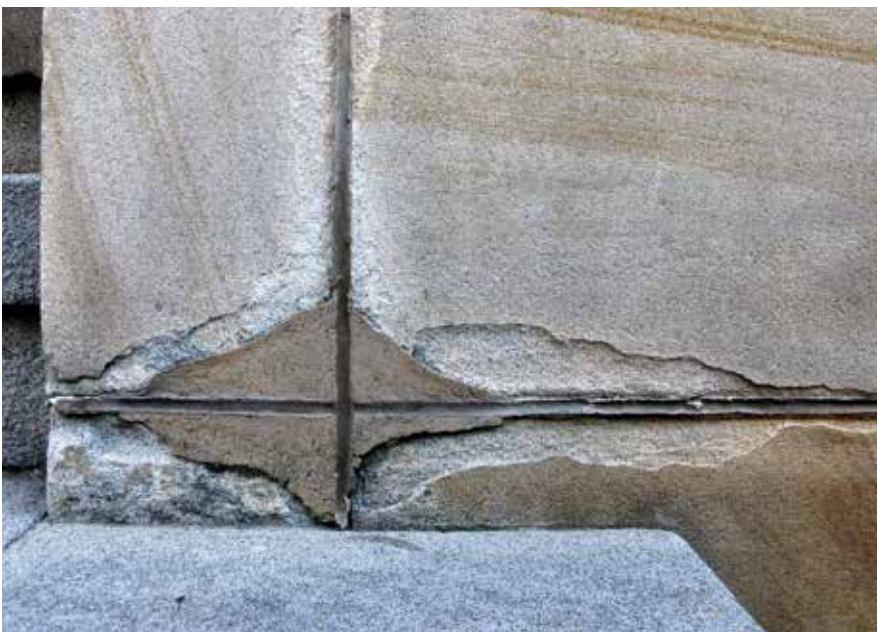
Figure 47: Inappropriate use of elastomeric sealant. Pointing the joints with an impermeable sealant has forced moisture to dry through the porous stones (rather than through the joints), resulting in salt attack decay to the sandstone. The damaged stones have been repaired with an equally impermeable patching material, forcing decay further through the sandstone.
