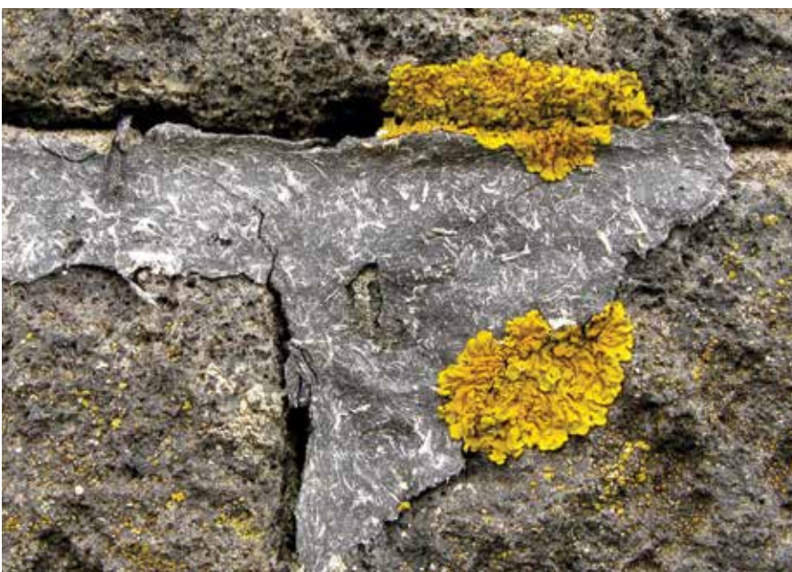
Figure 48: Old mastic sealant. The deteriorating sealant has pulled away from the adjacent stones, allowing water to enter the structure. Weathering of the sealant has exposed fibrous material which may be asbestos. Safety precautions must be taken when removing such materials (see Box 16 'Health and safety with mortars'). The bright yellow patches are lichens.
