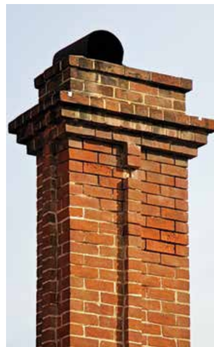
Figure 34: Which mortar? Because chimneys are more exposed, the initial response may be to use a stronger mortar than the original, but here the bricks are deteriorating, requiring a weaker, sacrificial mix (type 5).
