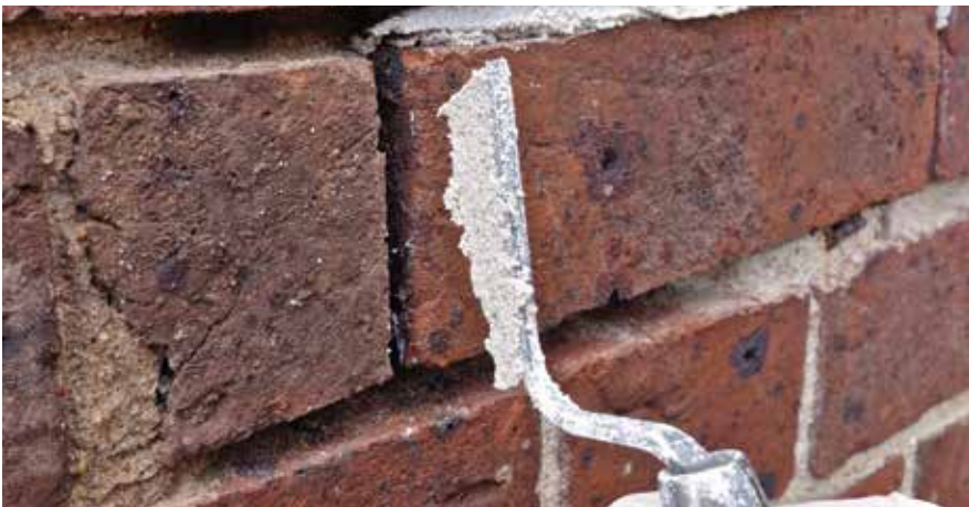
Figure 68: Filling a narrow perpend. Using a 4 mm wide trowel to place a thin wedge of mortar into a narrow joint. Careful placement with this technique removes the need to mask the face of the bricks with adhesive tape.
