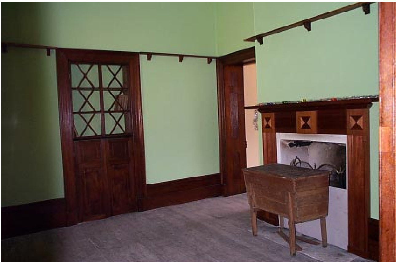
Current View of the conserved interior of the Royal Hotel Source: OCP Dec 2000
