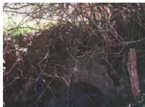
Stone culvert between Post Office and St. Bernard's Church is overgrown with vegetation Source: OCP April 2001
