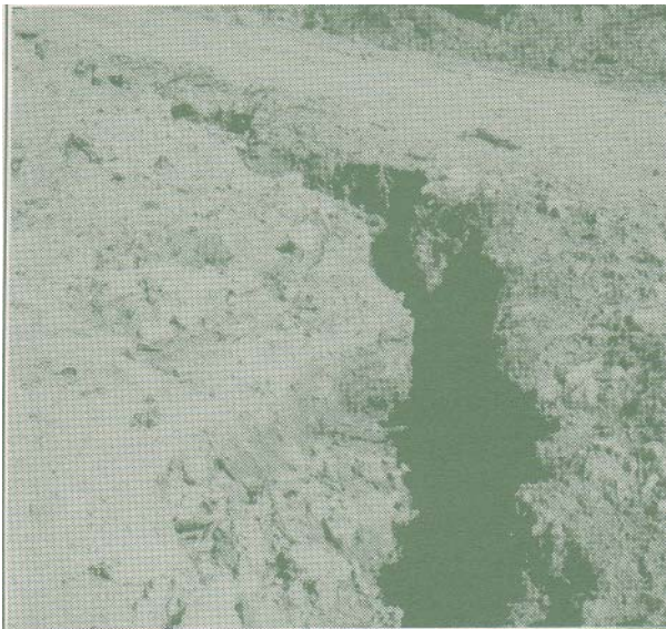
Gully erosion affecting track safety and generating sediment.
