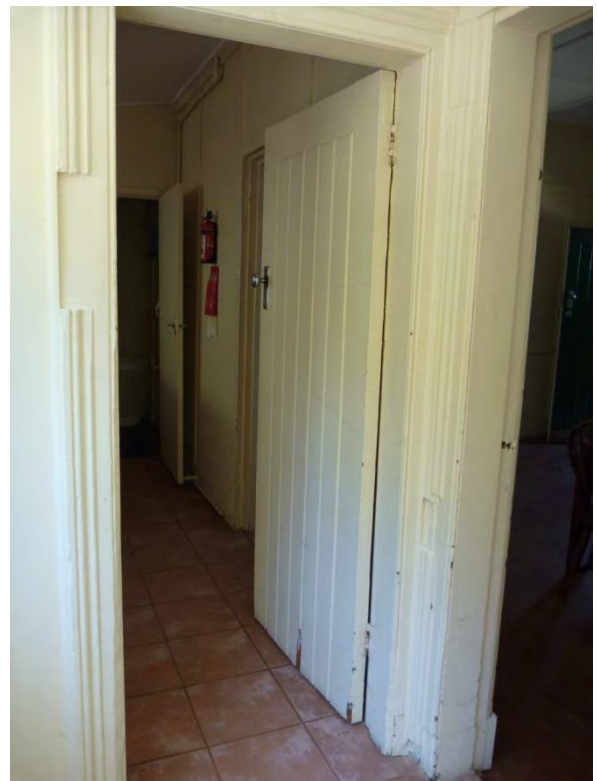
Figure 3.45 View from the rear enclosed verandah showing the remnant early/original architrave around the doorway to the rear wing. (Source: GML 2015)
