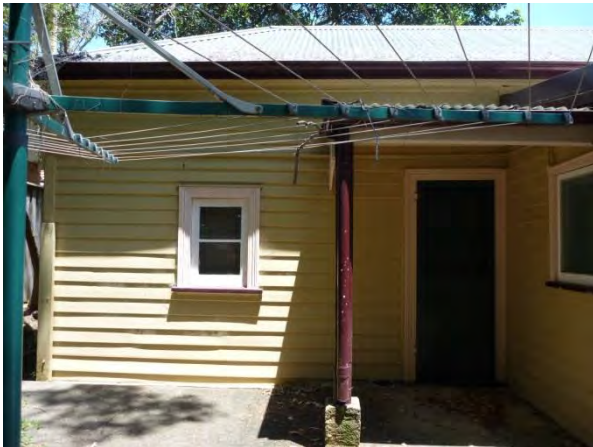
Figure 3.38 Original door and casement window to the northern wall of the easternmost bedroom. (Source: GML 2015)
