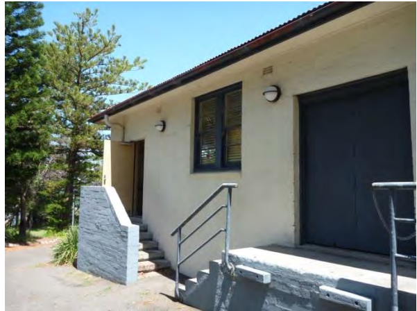
Figure 3.24 Two original entrances and double-hung sash windows on the eastern facade of the Armoury. (Source: GML 2015)
