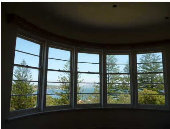
Figure 3.18 Timber-framed double-hung sash windows set out in a curve in the first-floor billiard room. (Source: GML 2015)
