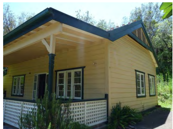
Figure 3.29 View of the Gap Bluff Cottage. Most windows are modern, simplified reproductions. (Source: GML 2015)
