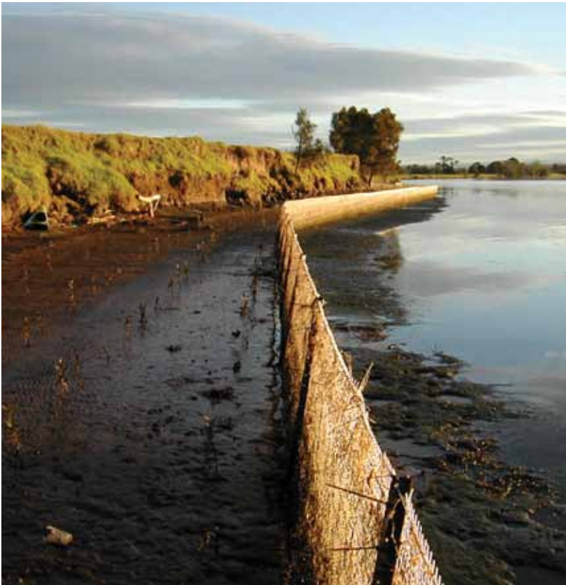
Figure 18: Mangrove seedlings planted in front of an eroding bank along the Shoalhaven River, with the use of temporary mesh fencing as a wave barrier and to protect establishing mangroves from debris. Photo—Allan Lugg, Department of Primary Industries.
