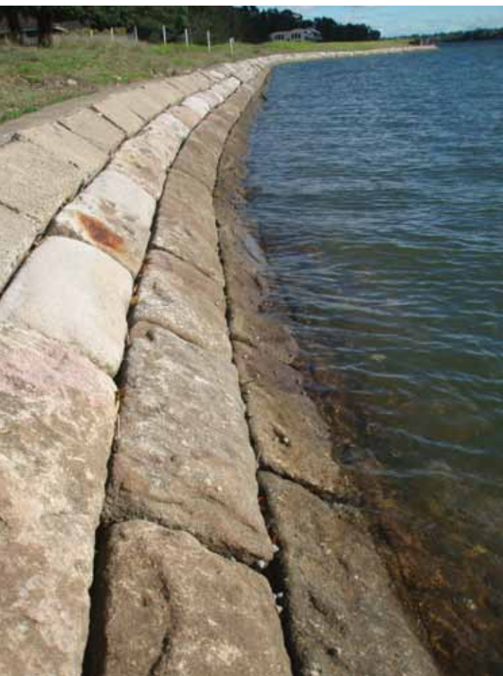
Figure 25: Examples of seawalls from Iron Cove, Parramatta River (left), and the Cooks River at Tempe (below) created without cement between the blocks to leave crevices, which provide valuable habitat.
