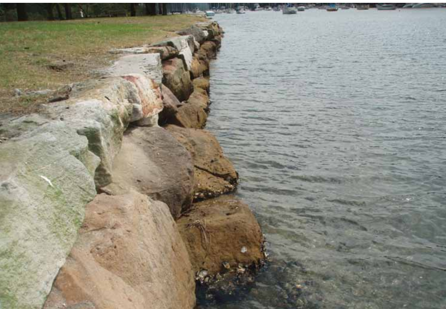
Figure 22: Example of a seawall made from boulders of various size and shape placed together without cement in McCarrs Creek, Pittwater.
