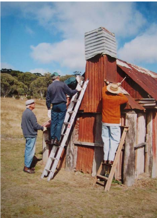
KHA working party repairing the chimney of the former Kitchen block/garage Source: Taylor family
