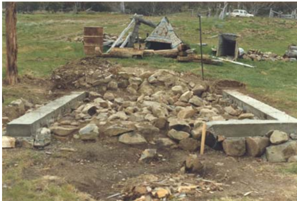
The Cheese Hut during the rebuilding, 1987. Note the concrete strip foundation and the stockpile of salvaged materials including stone. Source: NPWS Tumut
