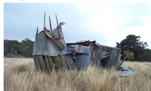
Collapsed slab hut in Yanunbeyan National Park
