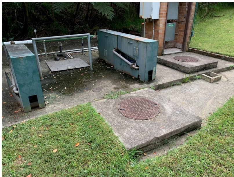
30 The sewage pumping station located on Wharf Road. Sewage is pumped to CP5 and then onto the neighbouring Australian Institute of Police Management and from there it to the municipal sewer system.
