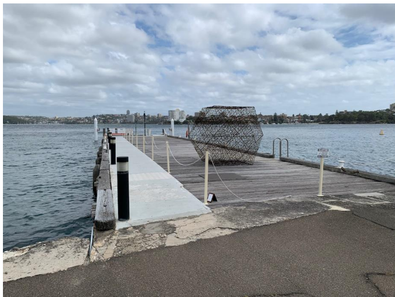
38 The Wharf - wooden sheeting had been placed on one side to manage trips and falls.
