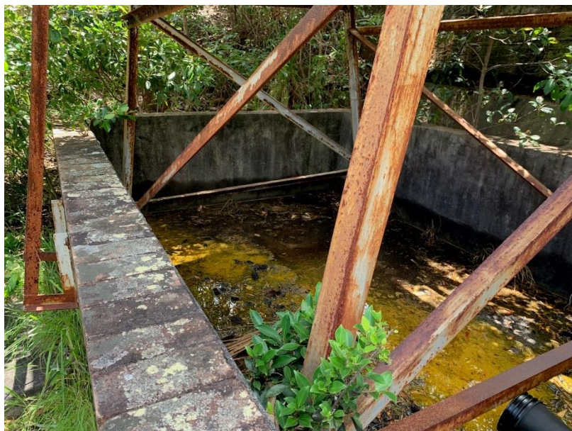
48 The bund to the former aboveground storage tank located opposite Building A18 Former Locomotion Shed was observed to contain a shallow layer of water and a diesel odour was noted coming from inside the bund.
