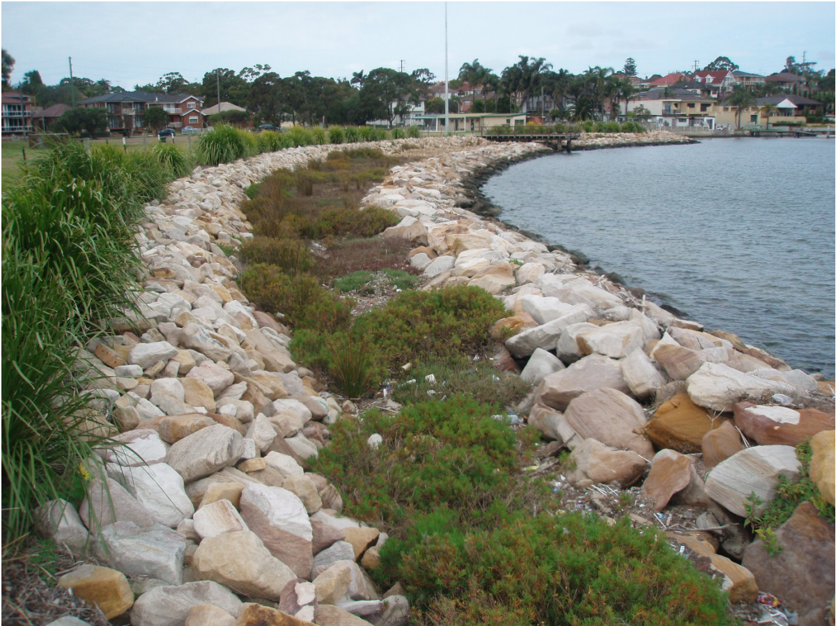
Figure B3.14 Seawall at Kogarah Bay showing step-type seawall with a bench of saltmarsh vegetation (Photo: D Wiecek/OEH)
