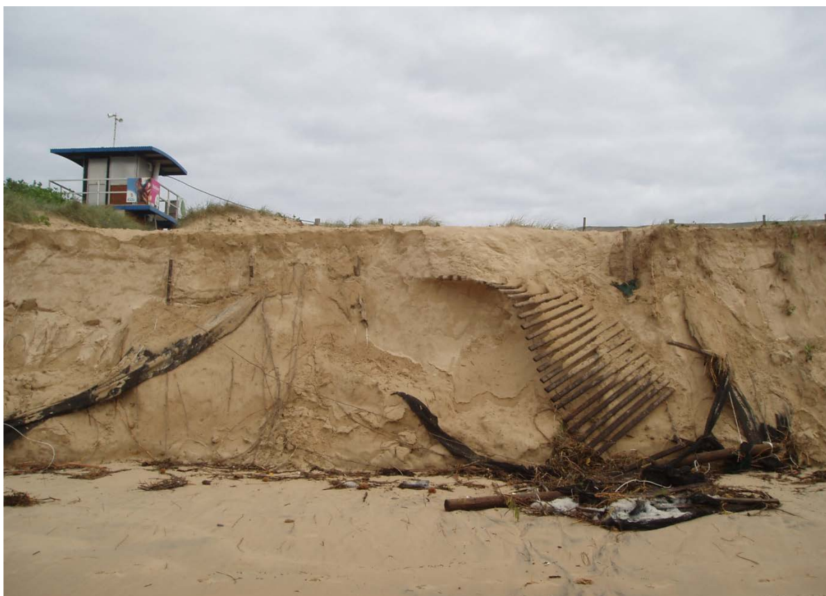
Figure B2.23 Risks to public safety from coastal erosion, Park Beach, Coffs Harbour (Photo: OEH)
