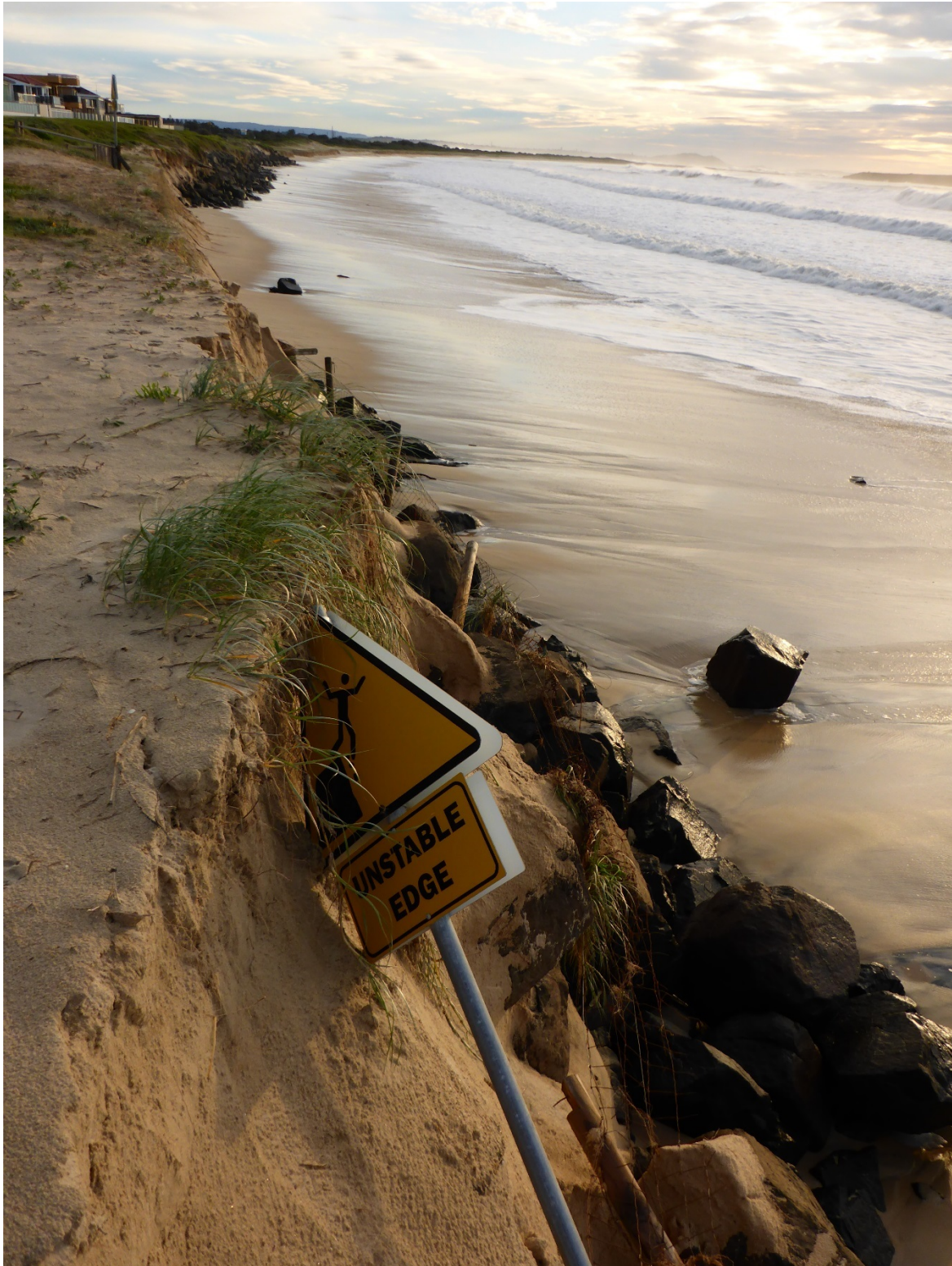
Figure B2.7 Storm damage to Warilla seawall, including loss of access control fencing and safety signage (Photo: D Wiecek/OEH)
