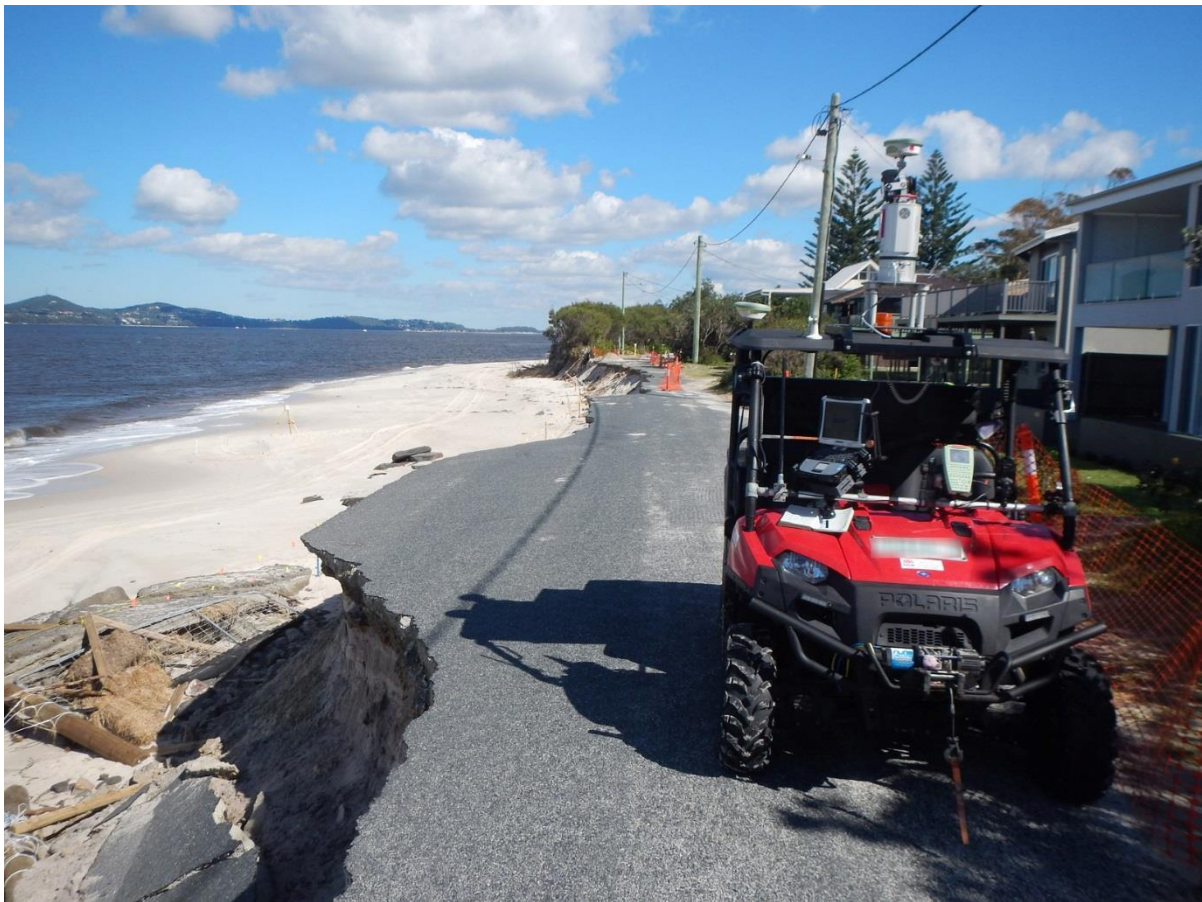
Figure A9 Road damaged by coastal erosion, Jimmy's Beach, Hawkes Nest (Photo: P Davies/OEH)
