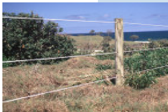
Figure 4.7b Bayco® fence, Angourie
