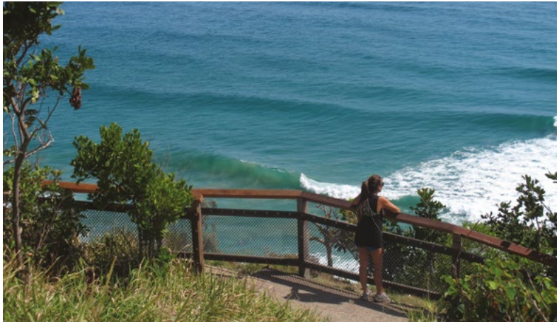
Figure 64 Existing balustrade on this section is new and in good condition (Context, 2016)
