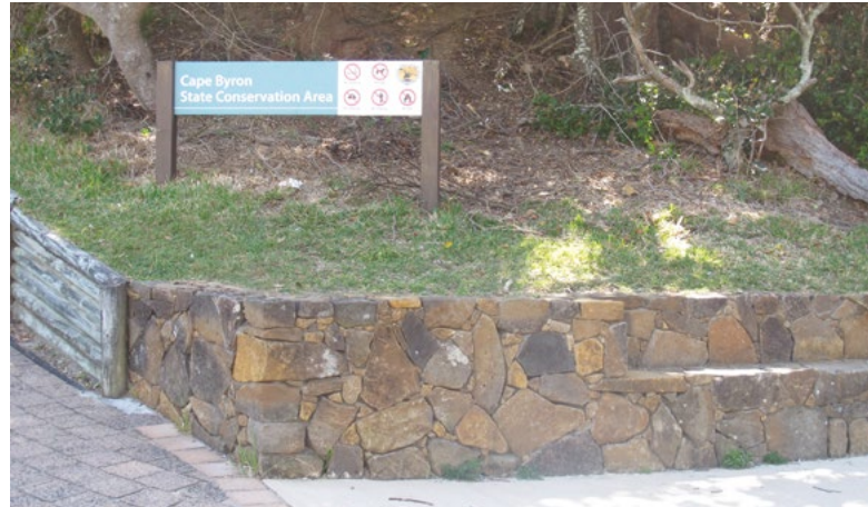
Figure 65 One of the new dry-stack walls already incorporated from previous plans (Context, 2016)
