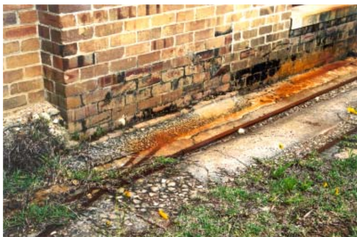
Figure 3.6.35 Rising damp to front wall of magazine No.14, 2001
