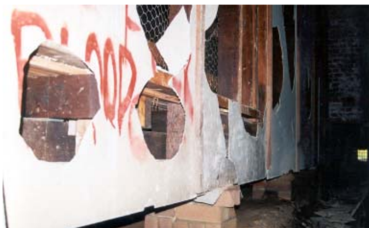
Figure 3.6.33 Damage caused by vandals to interior of magazine No.16, 2001
