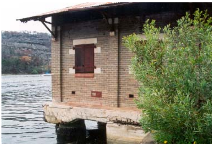
Figure 3.6.30 Suspended floor of receiving shed over water, note concrete corrosion, 2001
