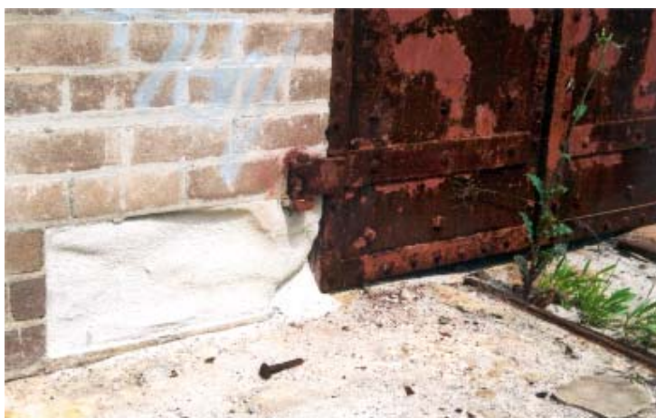
Figure 3.6.27 Erosion of sandstone anchor block of magazine, 2001
