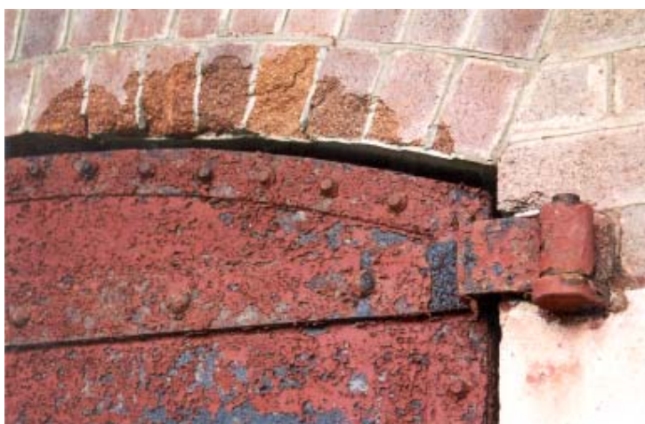
Figure 3.6.28 Corrosion to external iron doors of magazine, 2001
