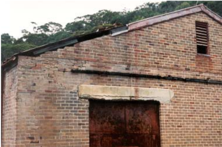
Figure 3.6.32 Cracking to magazine No.9, indicating subsidence, 2001
