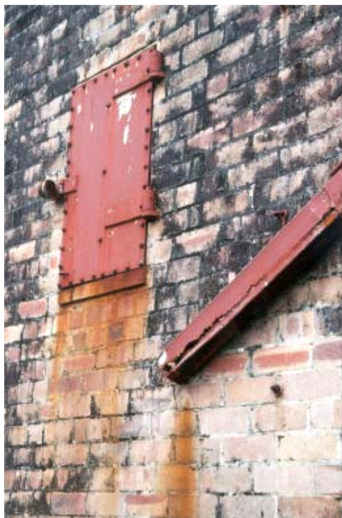
Figure 3.6.34 Water staining from shutters and downpipes to magazine No.16, 2001
