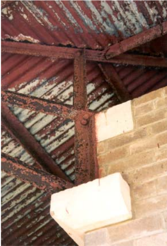
Figure 3.6.29 Corrosion and flaking paint of magazine roof, 2001
