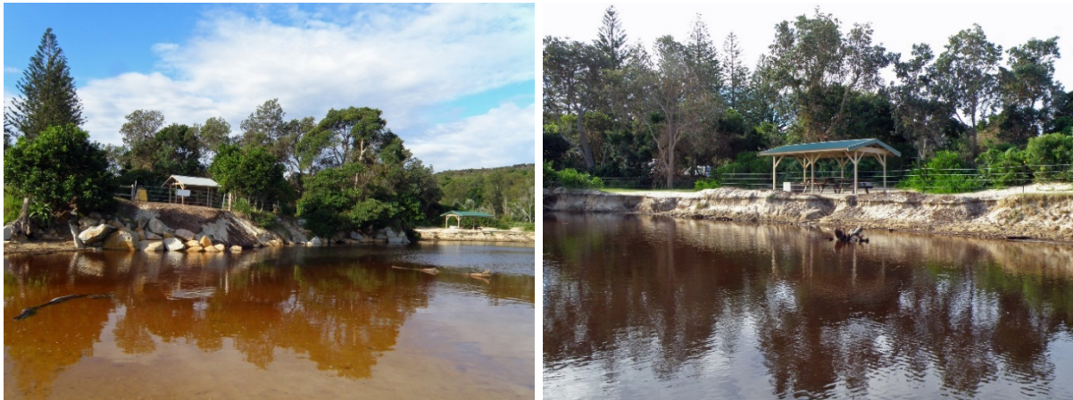
Photo 6 Stormwater runoff from Runaway Creek has caused erosion threatening built assets. Andrew Baker/DPE (2021).
