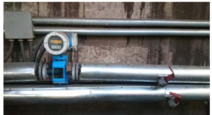
Figure 7 Water flowmeter. (Shutterstock)
