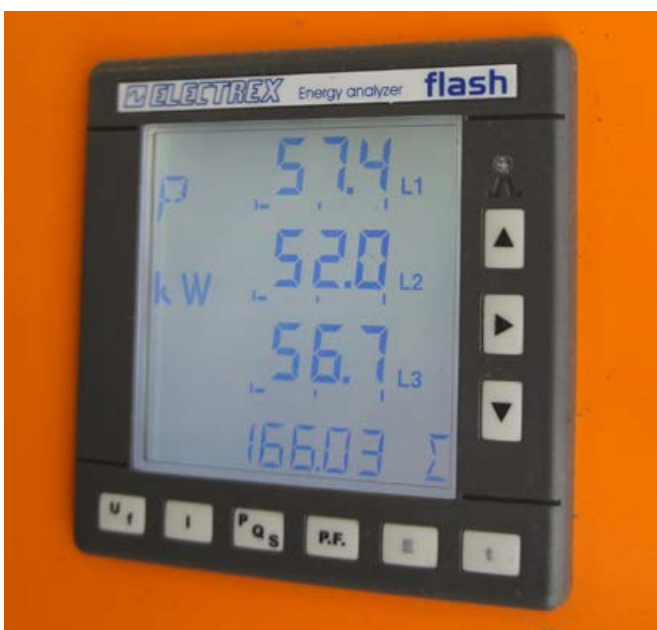
Figure 6 Electrical meter. (OEH)
