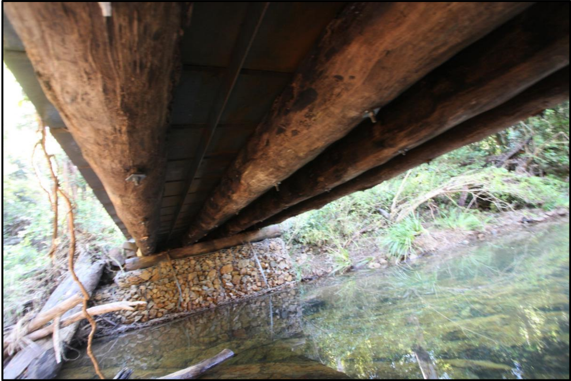
Figure 5: Budds Crossing Road Bridge deck girders and underside of the concrete deck, facing north.
