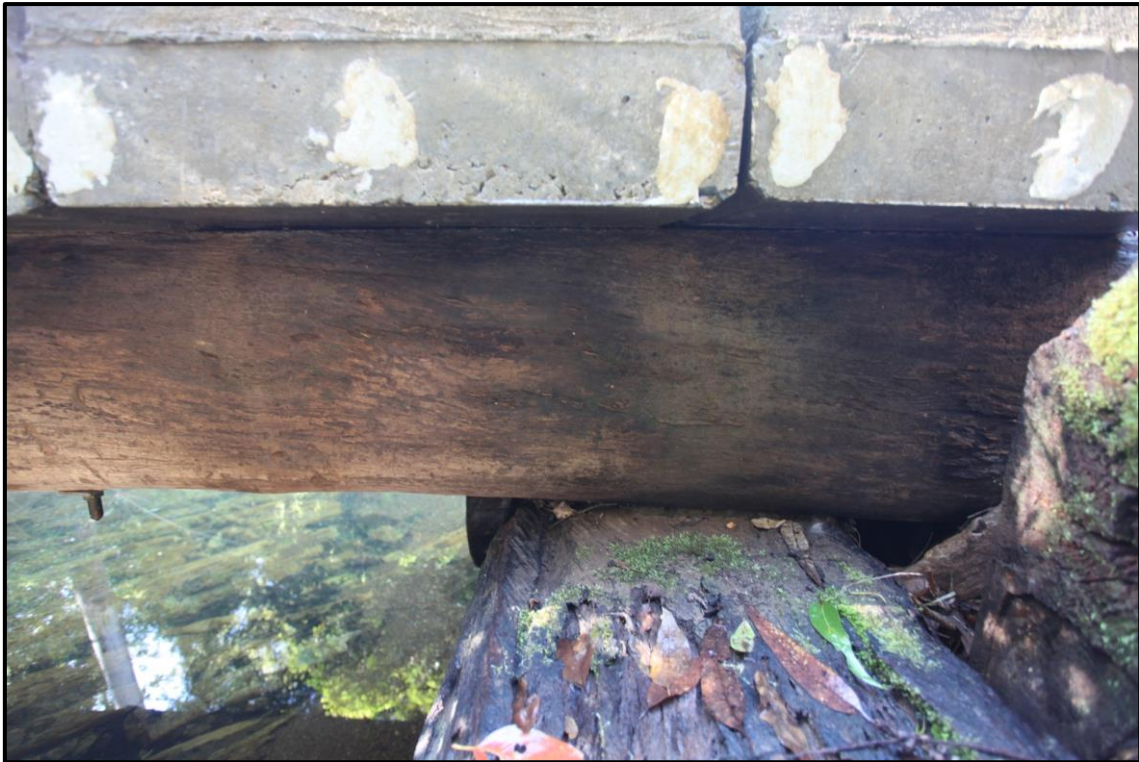
Figure 7: Cross section of the northern end of Budds Crossing Bridge, facing west.
