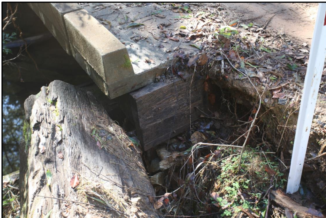
Figure 8: Relationship of the concrete slab deck to the southern timber abutment, facing north.
